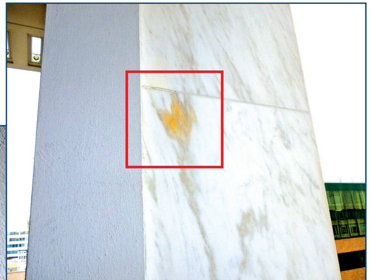
Figure 8 – Rust-colored staining observed at the ninth-floor intermediate joints.
