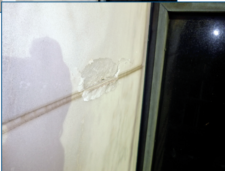
Figure 12 – Typical shallow spall observed at the edges of the marble fin panel joints.
