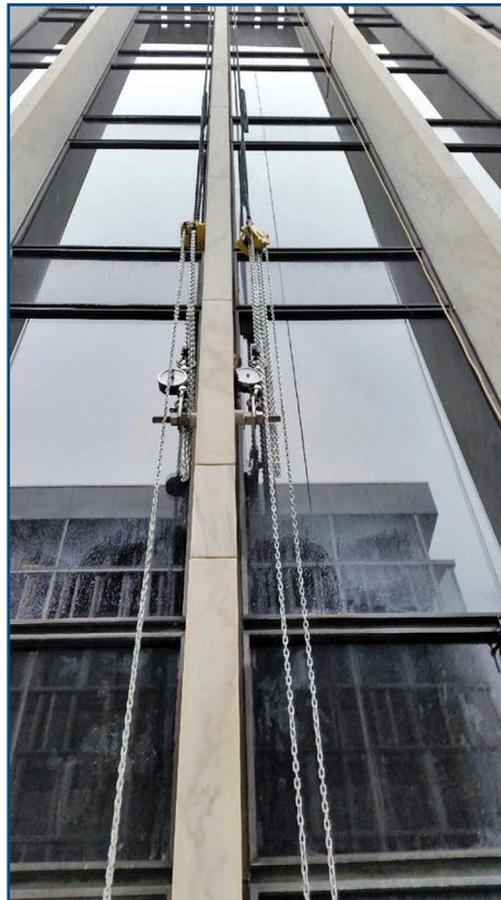
Figure 16B (left) – Trial installation of stone support system, which included a steel frame (Figure 16A), chain, chain hoists, tensioner, and chain anchored to steel dowels installed through the stone.
