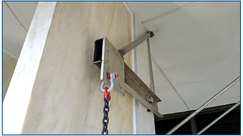
Figure 16A (above) – Custom-built steel support frame installed on both sides of panel and anchored into the concrete column and overhang.
