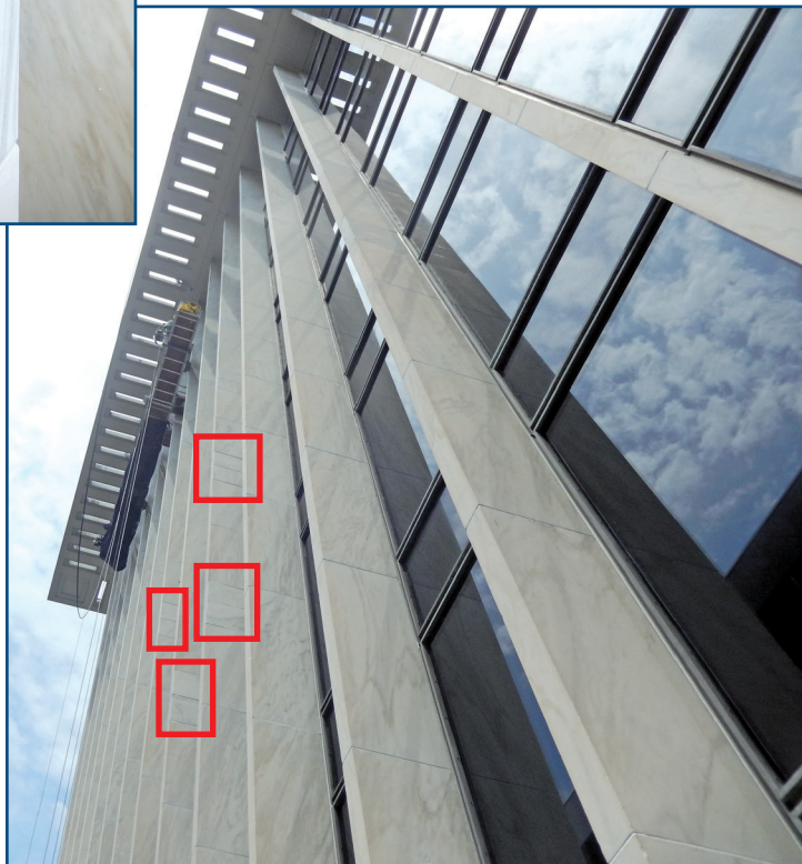
Figure 20 – Completed repairs of damaged marble fin panels at floorline and intermediate joints.
