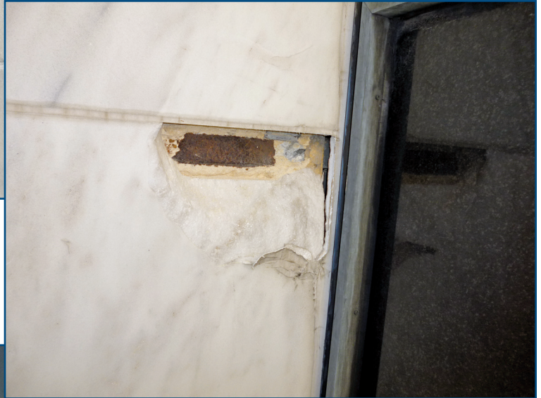
Figure 10 – Removed incipient spall at marble fin panel below the floorline gravity support. The steel bar of the panel support is corroded.
