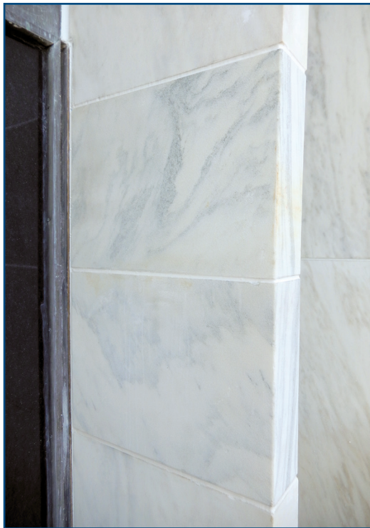
Figure 19 – Completed repair of damaged marble fin panels at a floorline joint (gravity support).
