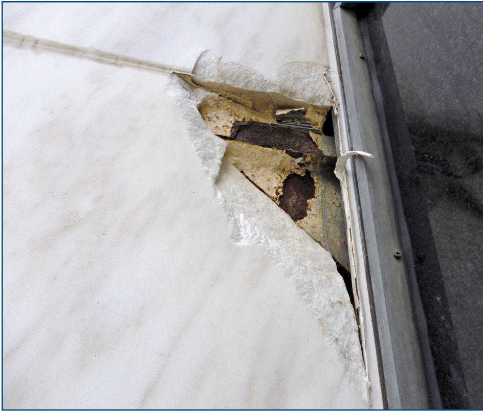
Figure 14 – Substantial corrosion observed on the steel bar and stiffener plate at the location of a removed incipient spall.
