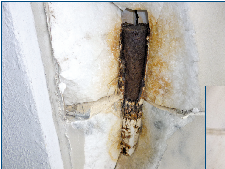
Figure 9 – Corroded dowel exposed by removal of a spall at ninth-floor intermediate joint.
