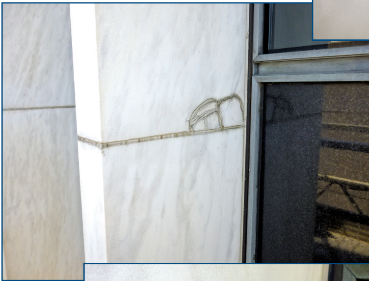
Figure 11 – Cracks and an incipient spall in a marble fin panel above a floorline joint previously repaired with sealant.
