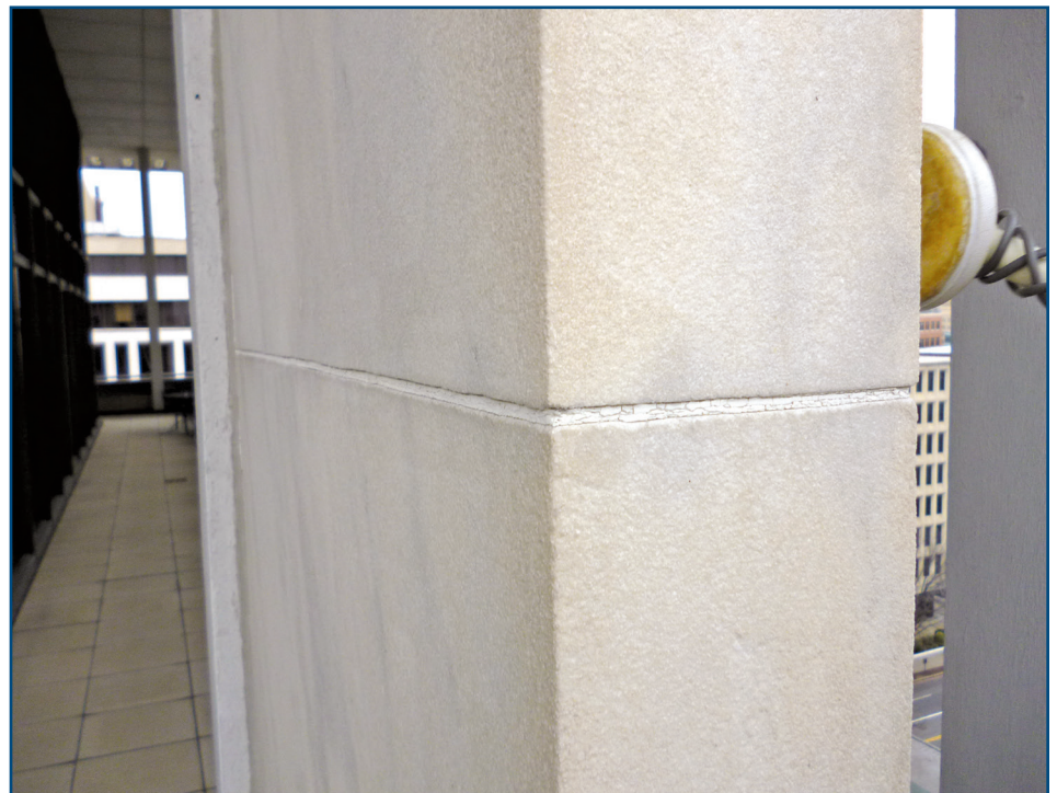
Figure 13 – Typical example of deteriorated sealant at a marble fin panel joint. The sealant was thinly applied over the existing mortar.
