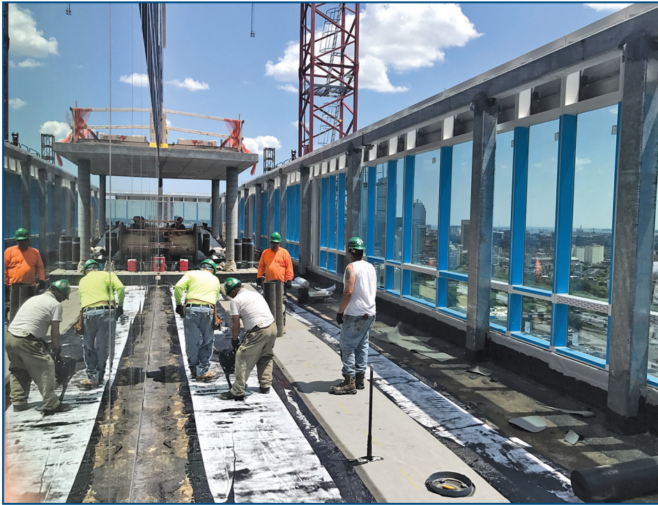
Figure 2 – The glass and aluminum curtainwall projects past the roof, forming a screen wall. Hot rubberized asphalt waterproofing is applied on a sloped concrete deck.
