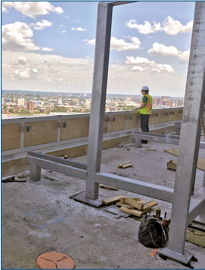
Figure 4 – Structural penetrations for screen walls and glass rails must be considered as part of the project’s energy conservation goals. A consultant takes in the great views from the soon-to-be-completed private cabanas.
