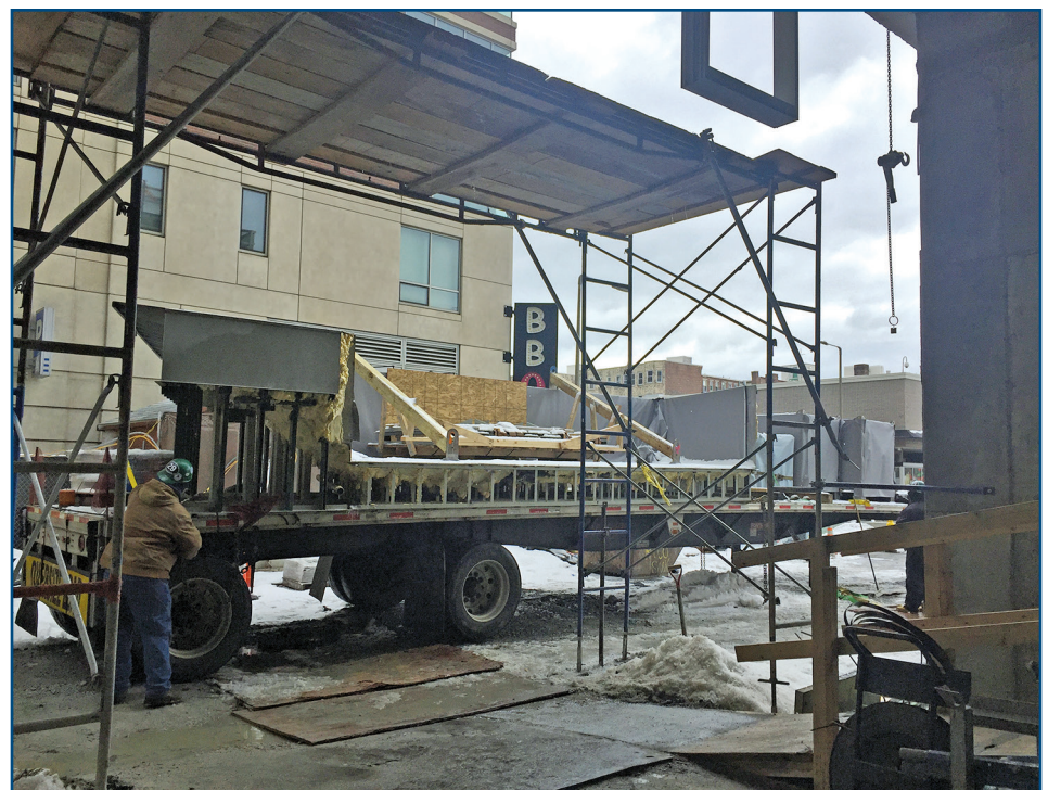
Figure 3 – Spray-foam insulation installed on underside of prefabricated pool shell. Photo courtesy of CBT Architects.
