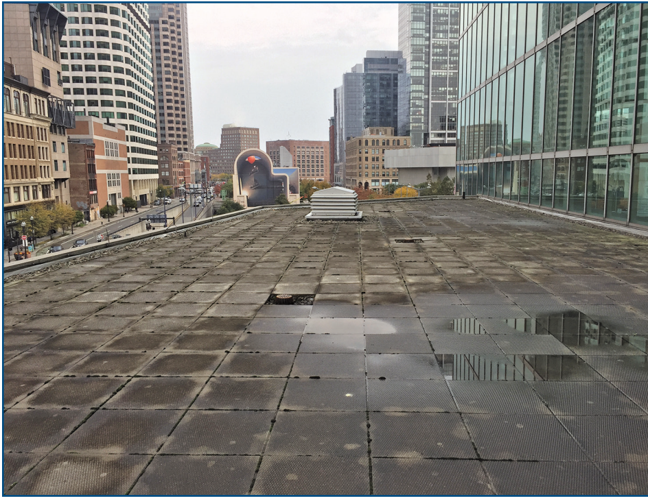
Figure 11 – Existing roof to be converted to useable space. Note the elevation of the curtainwall relative to the surface of the pavers.
