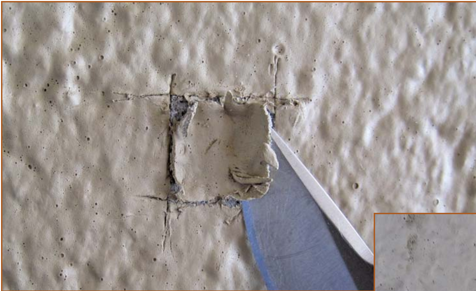
Figure 5 – A physical sample of the coating application is removed from the wall with a knife. The coating sample can then be easily measured via multiple simple tests.
