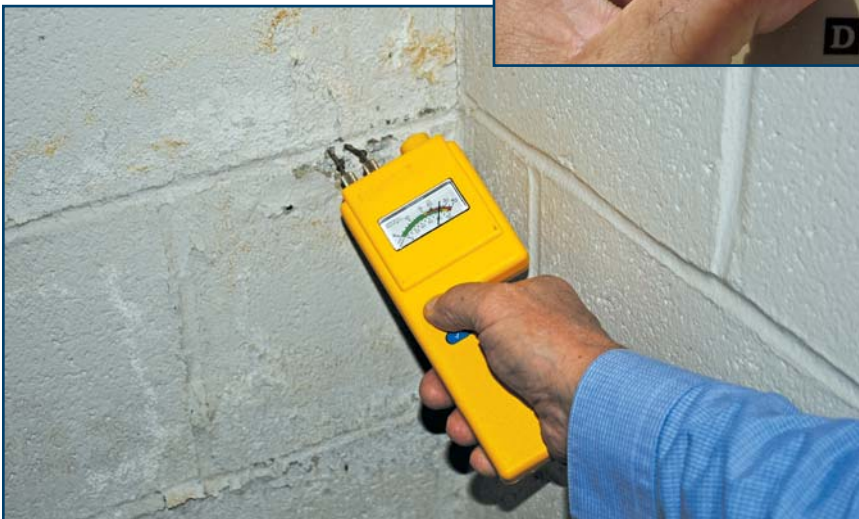
Photo 8 – Masonry nails are driven into mortar joints of CMU to assess the moisture below the surface.
