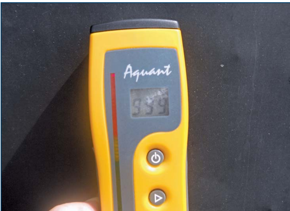
Photo 14 – Very high levels of moisture detected behind EPDM on a parapet.
