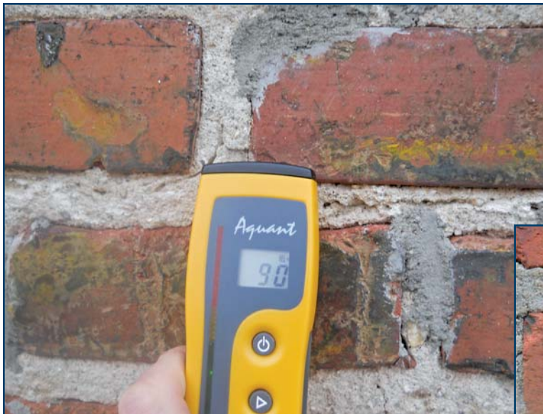
Photo 5 – Low (green) reading on mortar.
