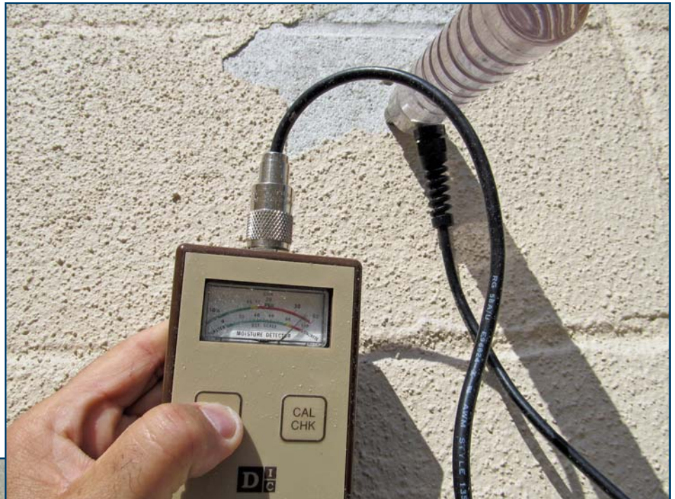
Photo 9 – Conductivity meter with 4-in. probes inserted into the block cell. Instrument reading shows that the insulation is wet.
