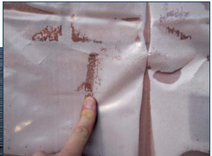
Photo 4 – Moisture visible beneath plastic.
