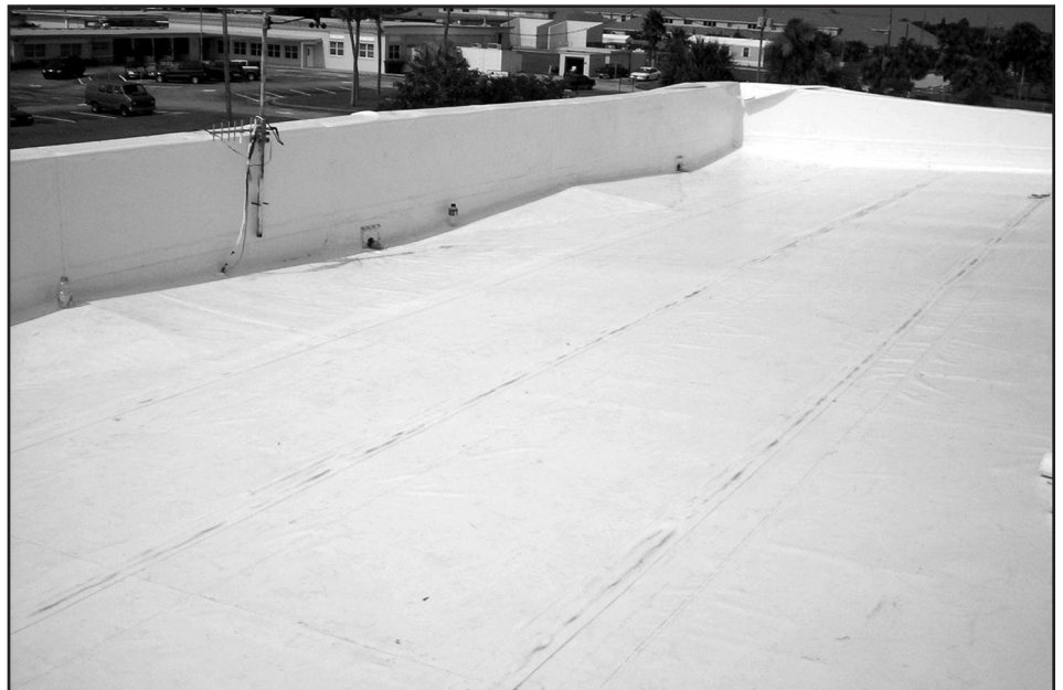
Photo 17 – This school had a mill-finish Galvalume® structural panel typical for a preengineered metal building.
