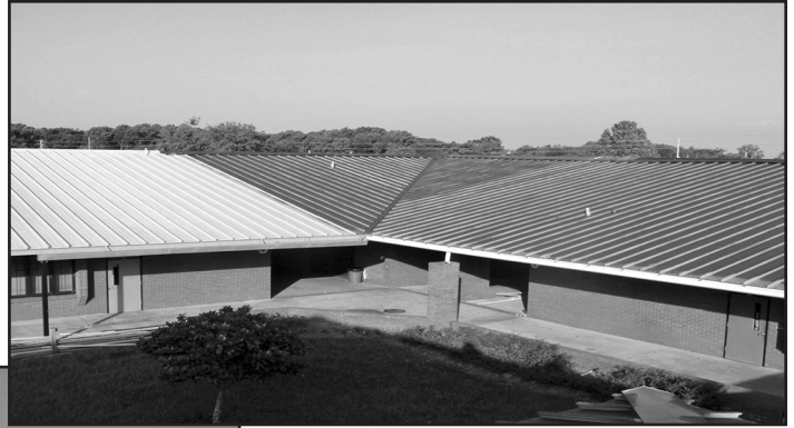
Photo 13 – Just prior to the coating application with the dead-level valley and ventilation cupolas eliminated.
