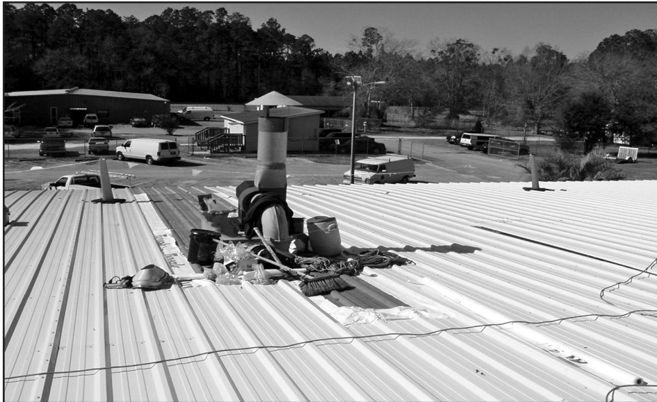
Photo 3 – A replacement system that seems to be unique to utility panels with exposed fasteners is overlaying an existing metal roof system with a nesting panel system.
