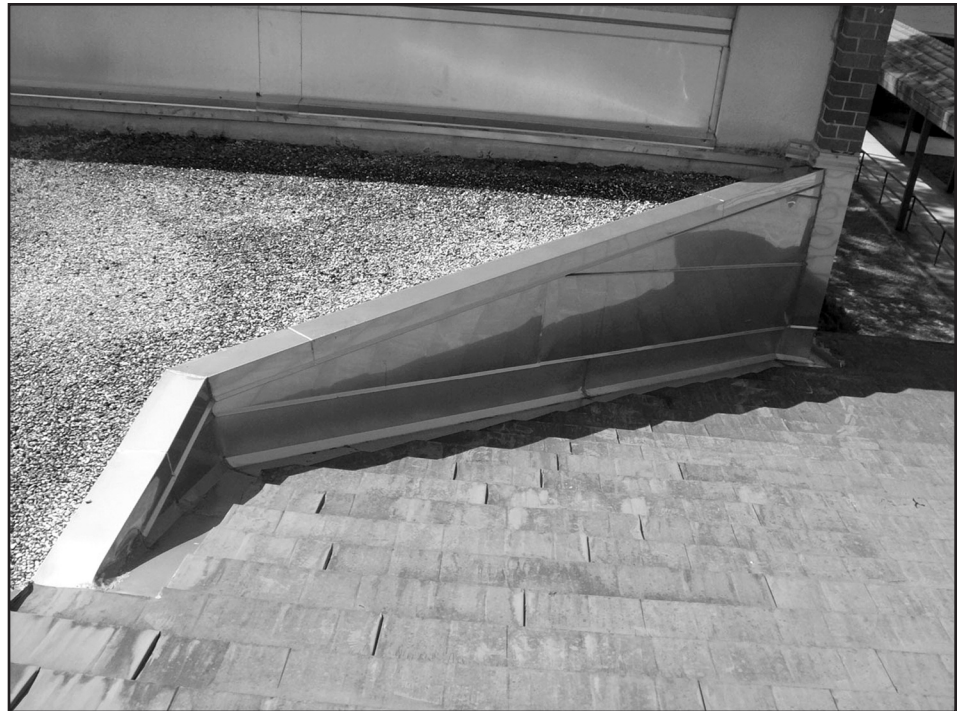
Photo 9 – Roof leaks were widespread throughout the field of the roof, but primarily at some angle walls, against and along which several roof areas drained.
