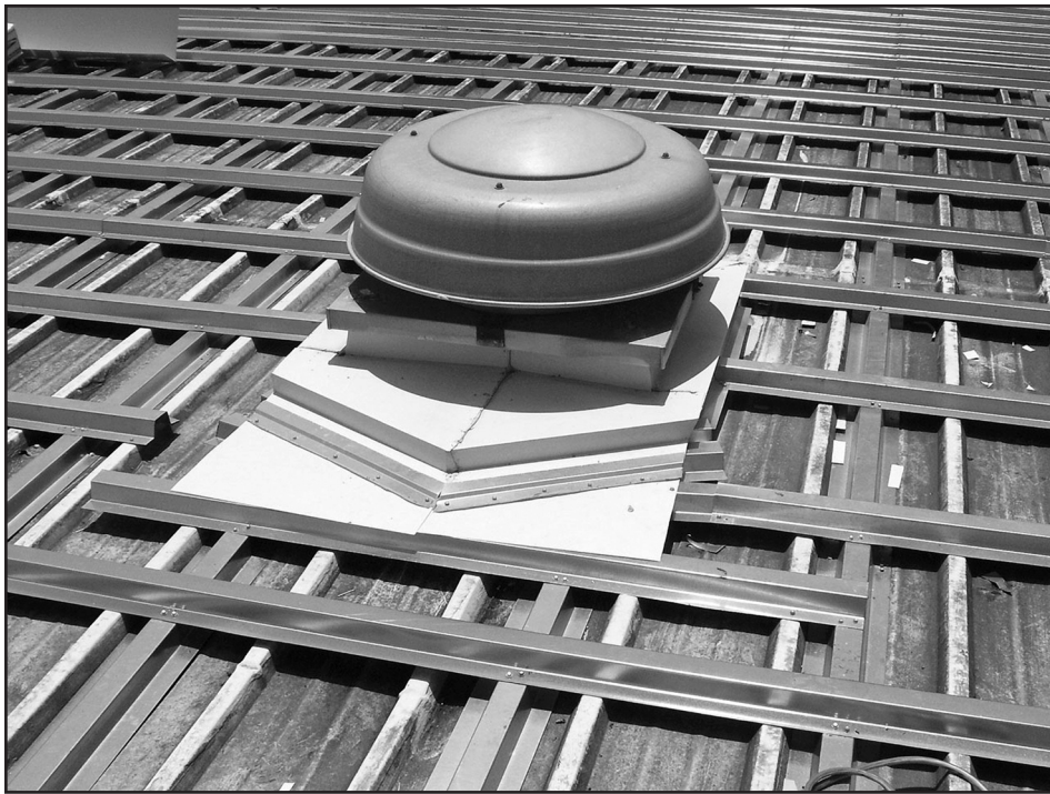
Photo 6 – This pre-engineered structural metal roof system over purlins incurred storm damage during Hurricane Charlie.
