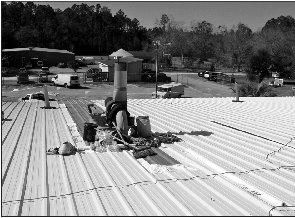
Photo 8 – The darker existing metal roof panel can be seen downslope of the exhaust fan; some building wrap is seen along the edge of the new white roof panel that has been installed.
