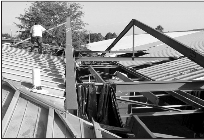
Photo 12 – The new framing used to extend the existing rooflines and eliminate this problem valley.
