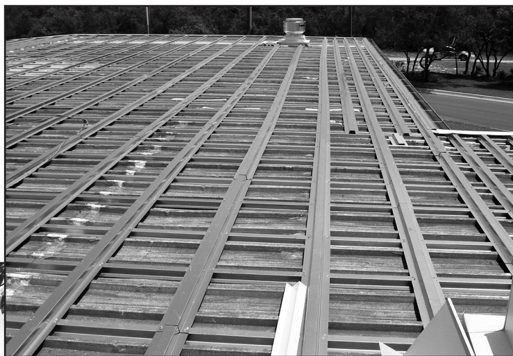
Photo 2 – In this double furring system, the first layer of furring runs up the roof slope and a second layer of furring runs across the roof slope.
