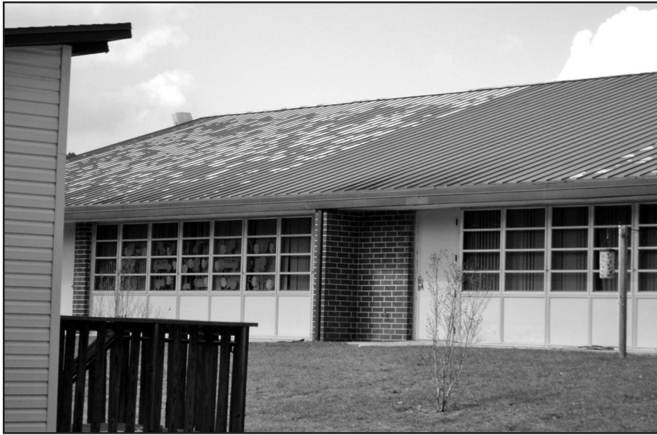
Photo 10 – This architectural standing-seam metal roof with a snap-on seam cap was experiencing water intrusion problems, primarily along an angled wall flashing.
