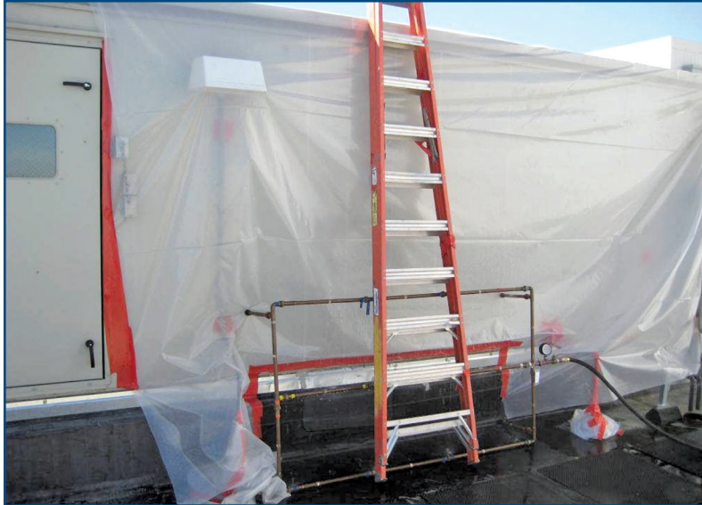
Figure 7 – Using an ASTM E1105 spray rack to test base of unit flashing.
