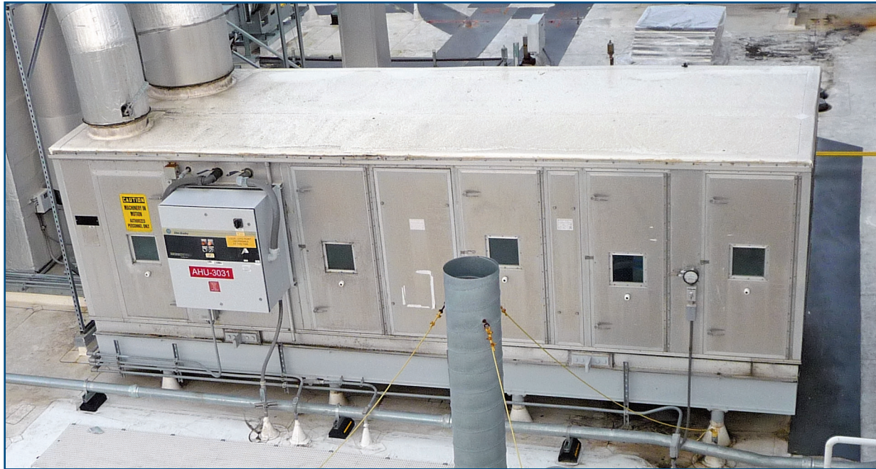
Figure 4 – AHU mounted on posts.
