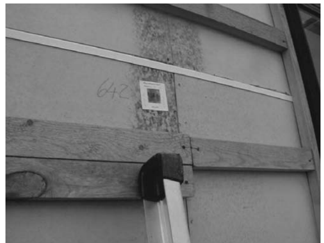
Figure 1 – Example of a ventilated façade with mold growth on the wind barrier (made by gypsum boards). Often mold growth in façades is due to water penetrating behind the cladding without being drained out (fast enough).
