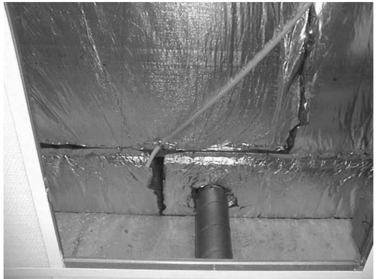
Figure 5 – Vapor barrier with leaks at joints and pipe penetration in a school. The entire school was built in the same way. The consequence was that there was massive mold growth in all roofs and that a major renovation was necessary to remove the mold.
