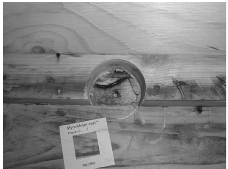
Figure 3 – Roof element in a new school with massive mold growth. The roof elements are prefabricated and meant to be sealed immediately after assembling. Lack of sealing, however, leads to penetration of water and eventually mold growth. The renovation included opening of the prefabricated elements, removal of insulation, and cleaning of the wooden surfaces in the elements. Afterwards, the elements were restored with new insulation and vapor barrier.
