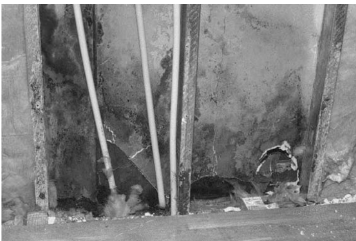
Figure 2 – Severe attack of mold on the backside of a gypsum board partition in a bathroom due to lack of a watertight membrane (the wall was tiled directly on the gypsum board).
