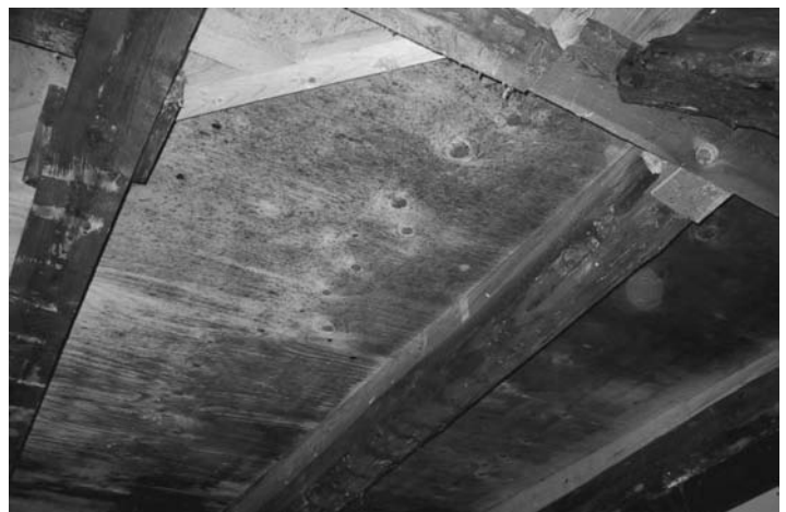
Figure 7 – Mold growth on plywood substrate for roofing felt in a ventilated roof due to sub-cooling caused by radiation to the sky. Plywood is more vulnerable to mold growth than boards, probably due to the treatment during production.
