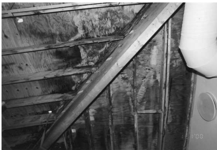
Figure 4 – Mold growth and deterioration of plywood in a sloped roof made from wood-based elements assembled in situ. Due to leaks in the interior joints between elements in the corners - and consequently also leaks in the vapor barrier – humid air has penetrated into the construction, where it condensates on the cold surfaces above the insulation.
