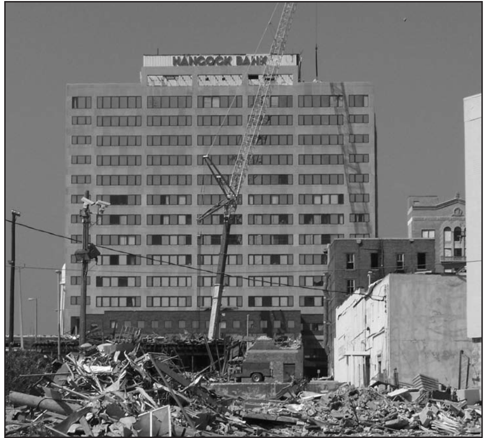
Figure 1 – Characteristic aggregate or small projectile impact damage to glazing in a wind-borne debris region on Hancock Bank Building, Gulfport, MS, caused by Hurricane Katrina (photo by M. Fischer).
