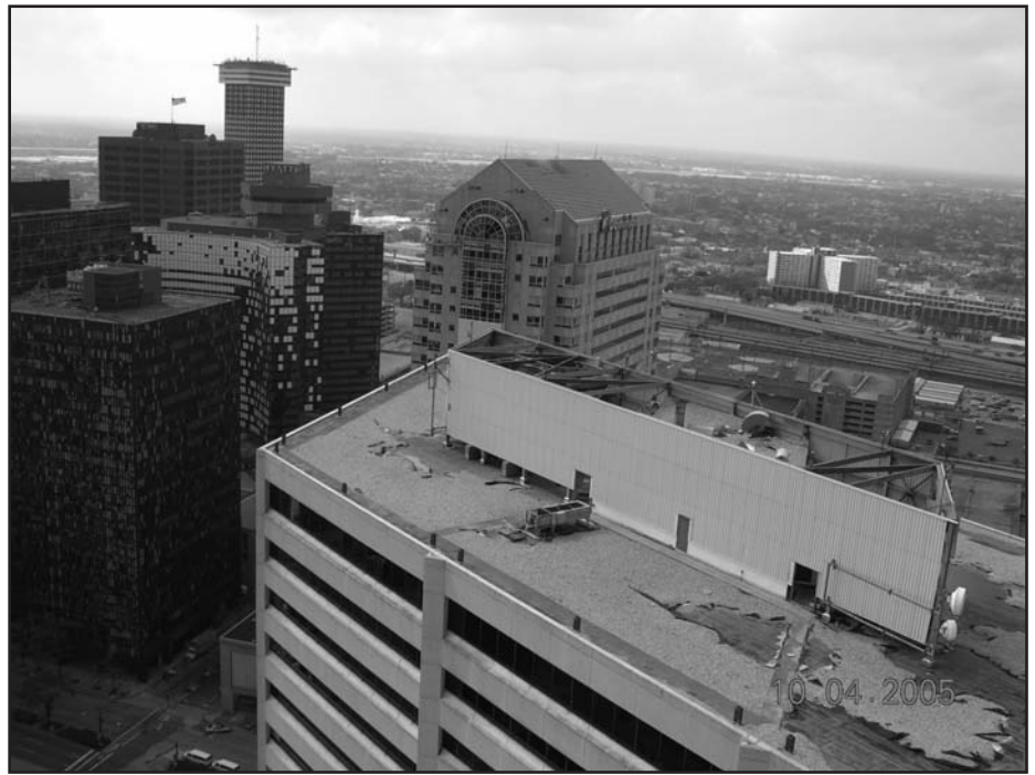
Figure 3 – Aggregate scour and blow-off from a “noncompliant” aggregate-surfaced roof in Hurricane Katrina in 2005 (photo from FEMA 549).
