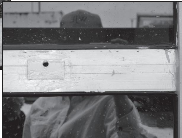
Figure 27 – Modified weepholes at other intermediate horizontal mullions.
