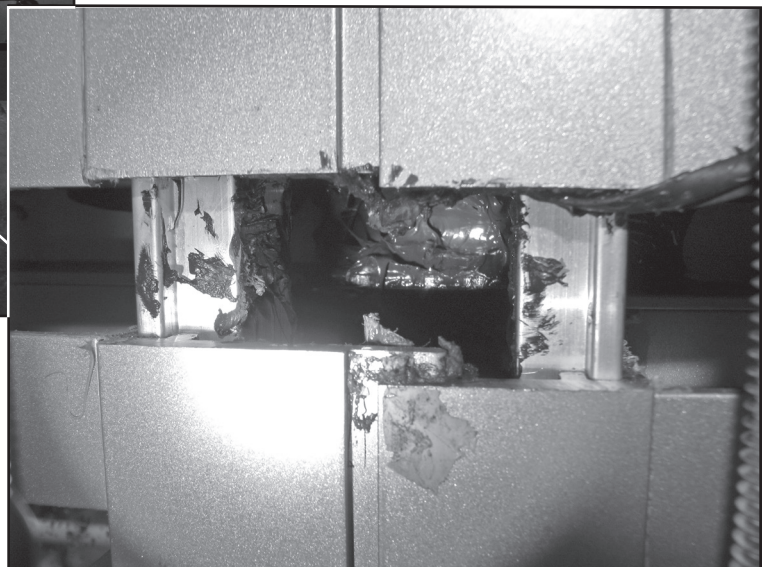
Figure 22B – Close-up of additional seal at hollow two-piece mullion stack joint condition.
