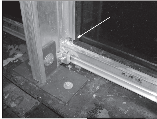
Figure 24 – Prematurely terminated interior glazing stop.
