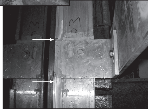
Figure 25 – Discontinuous interior glazing stop at mullion anchor.
