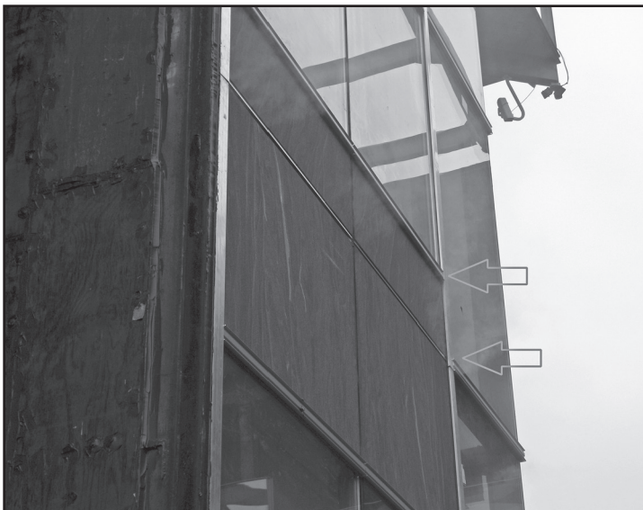
Figure 18 – Air exfiltration observed with smoke bomb and pressurized chamber.
