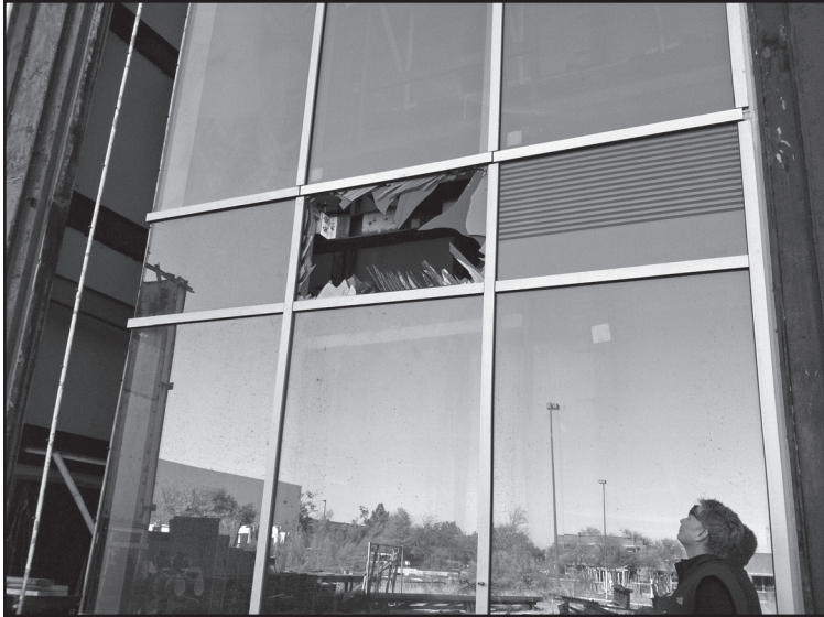
Figure 14 – Glazing breakage during 150% negative structural load testing.
