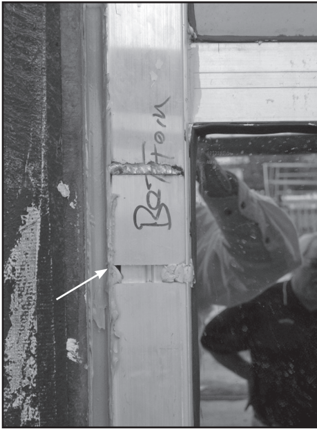
Figure 28 – Alignment plate at the face of the splice joint prohibiting proper field sealant installation.
