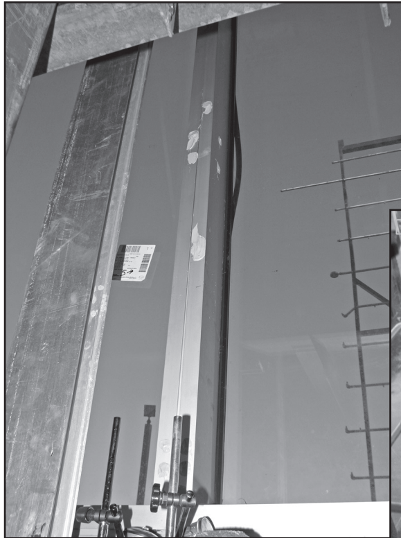
Figure 9 – Partial deglazing of vision unit due to excessive deflection of two-piece mullion for unitized curtain wall.
