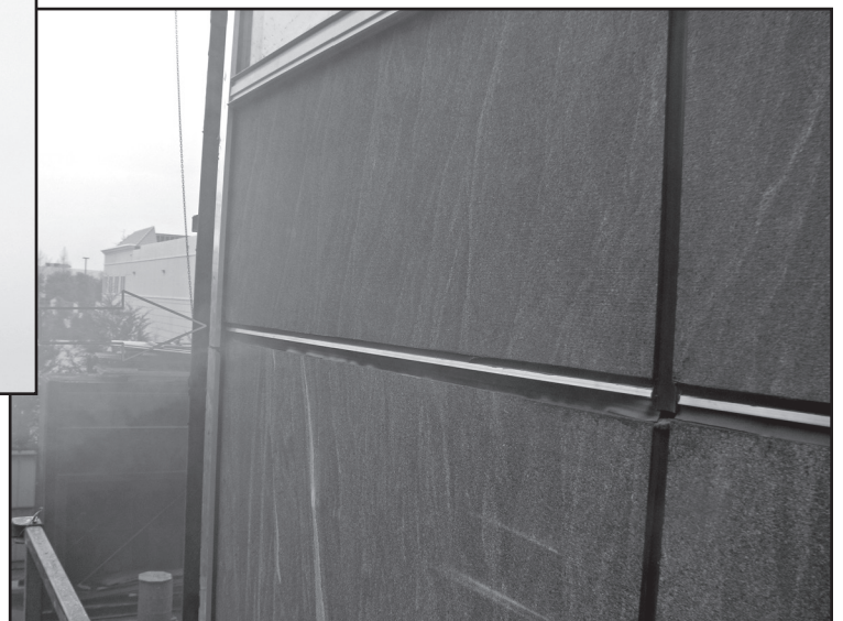
Figure 19 – Air exfiltration observed with smoke bomb and pressurized chamber.
