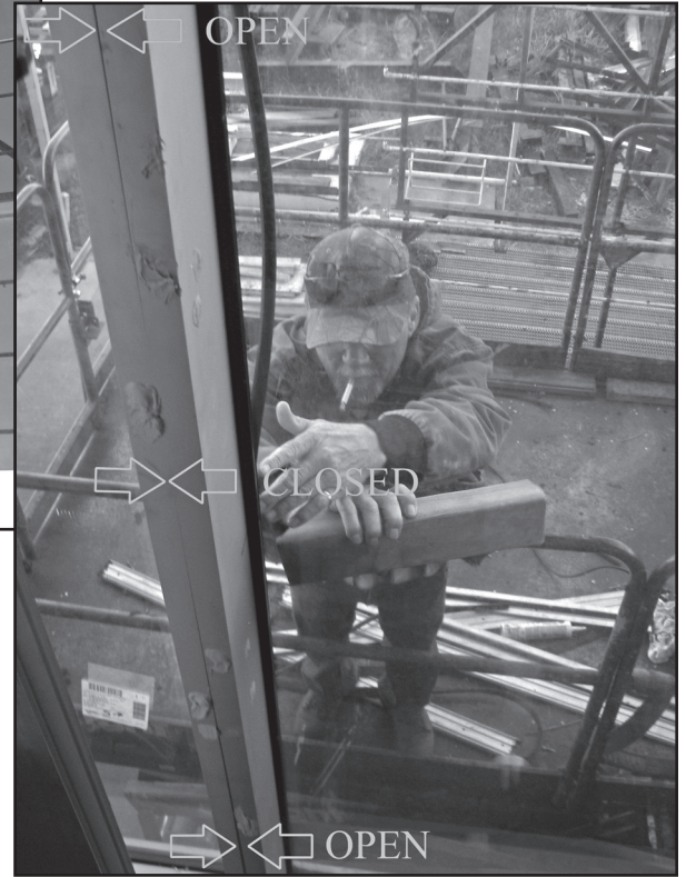
Figure 10 – Rolling of two-piece intermediate mullions and partial deglazing of IGU following negative-pressure structural testing.
