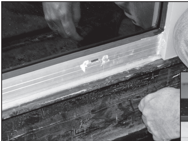
Figure 26 – Rectangular weepholes at base sill track.
