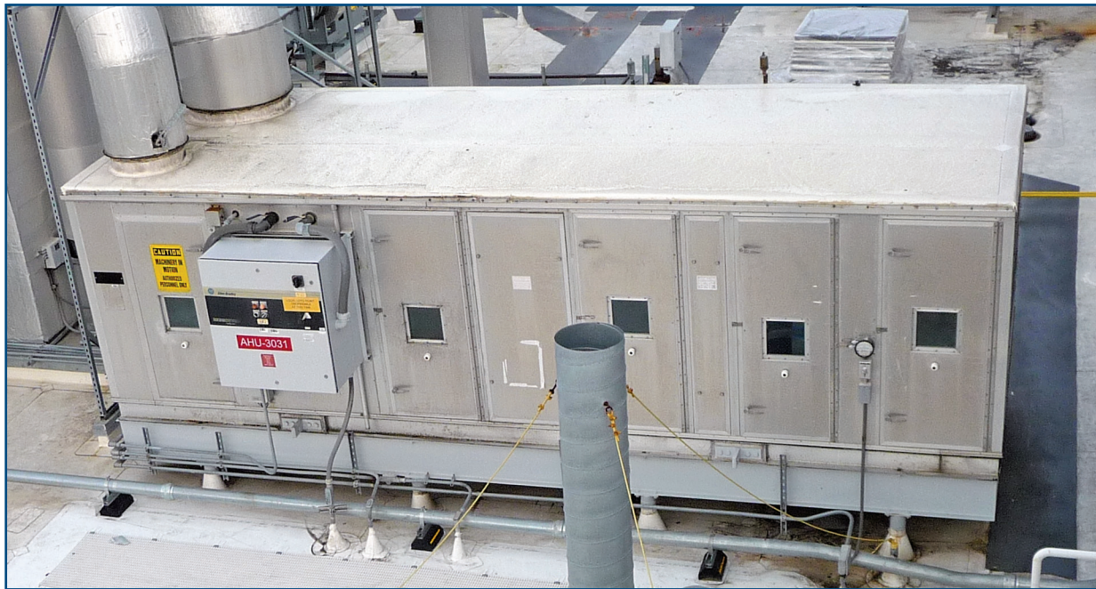
Figure 4 – AHU mounted on posts.
