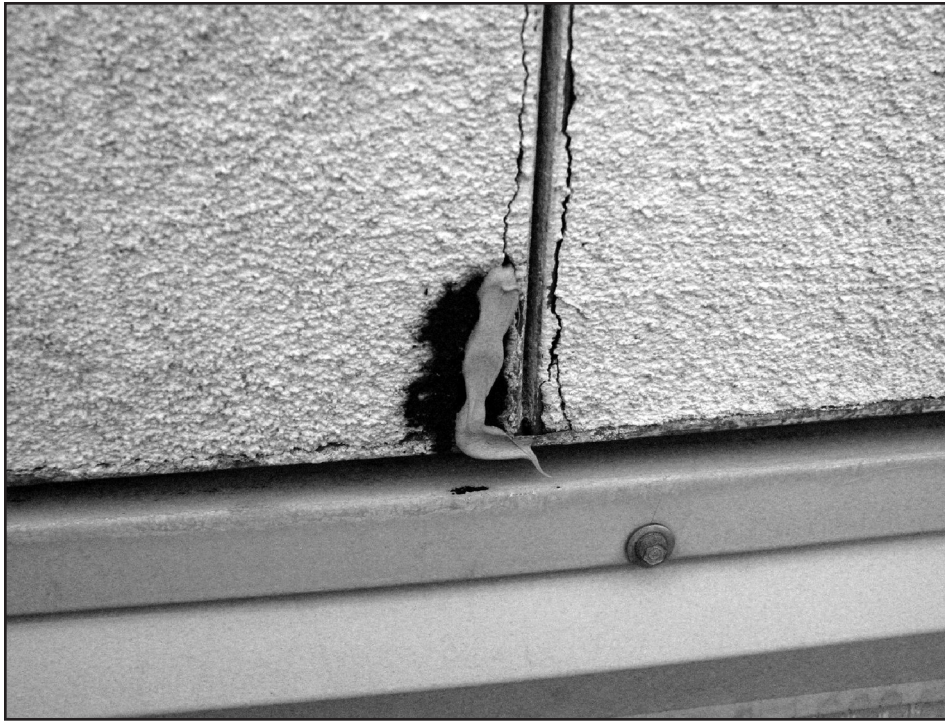
Photo 6 – Does this condition require further investigation?
