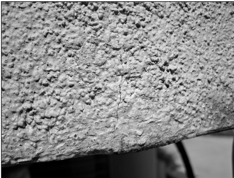
Photo 5 – Efflorescence and corrosion staining emanating from stucco cracks.
