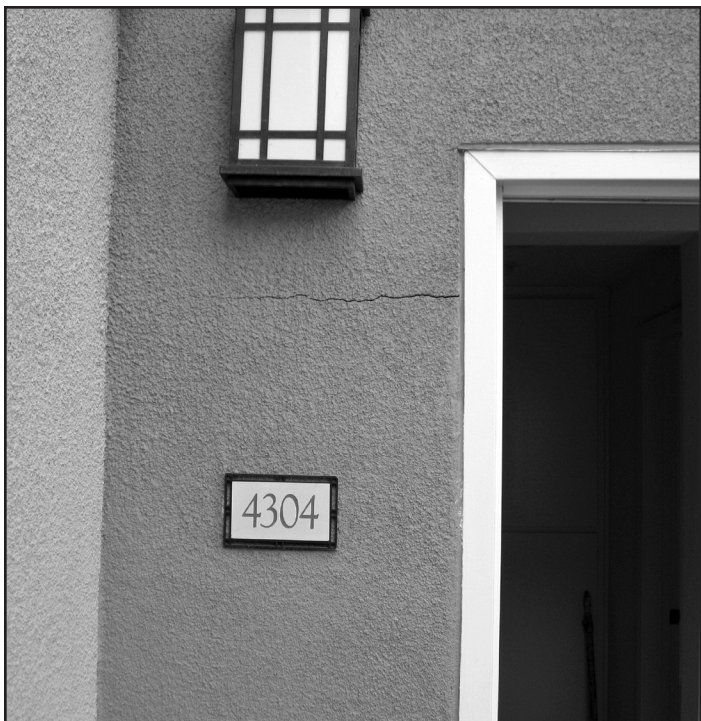
Photo 7 – Crack at entry door.
