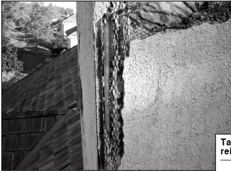
Photo 4 – Corroded metal lath.
