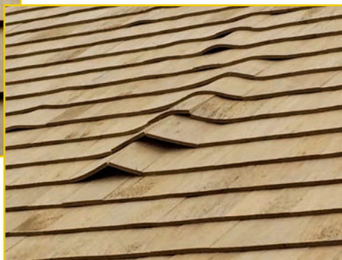
Photo 14 – Buckling due to improper keyway spacing.
