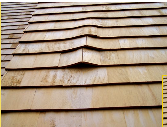
Photo 13 – Buckling due to improper keyway spacing.
