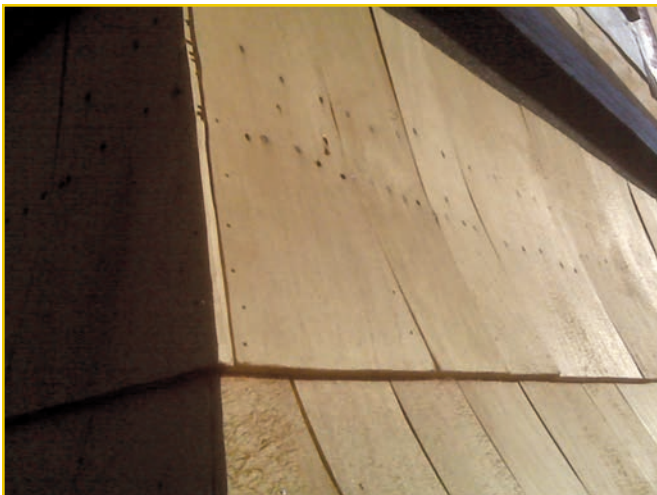
Photo 8 – Far too many fasteners on this application.
