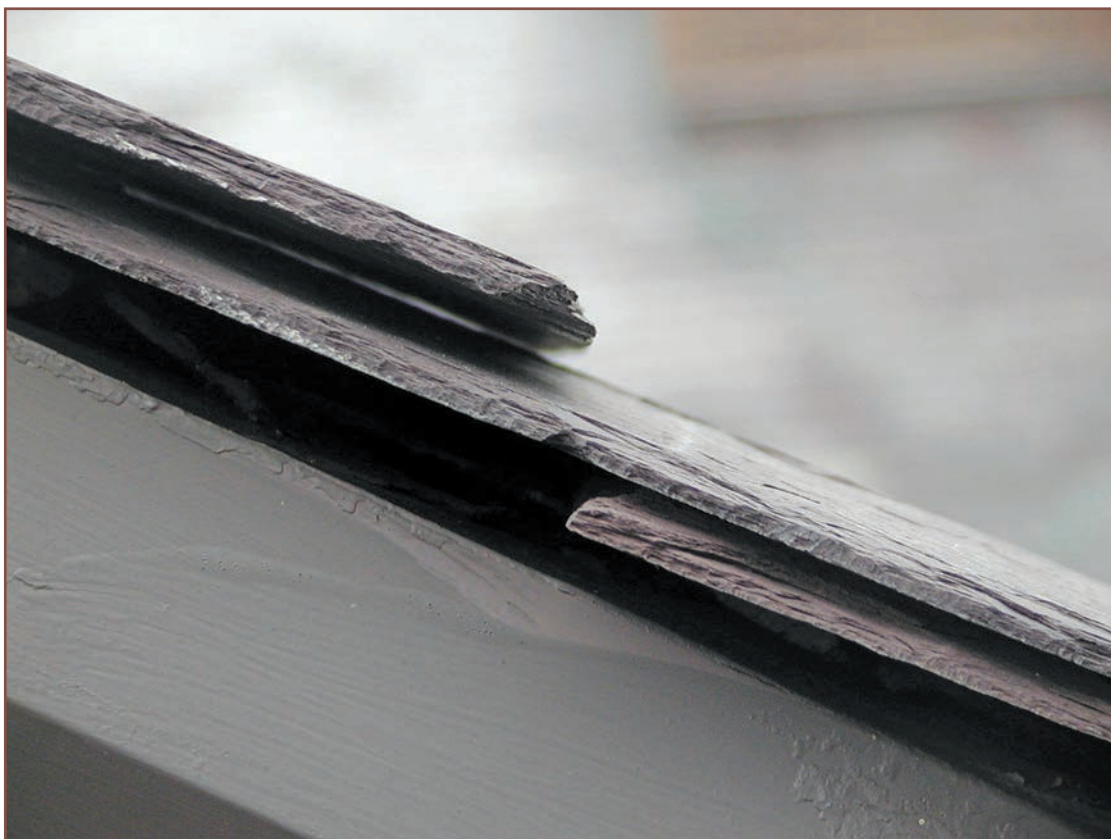
Figure 3 – Improper head laps.
