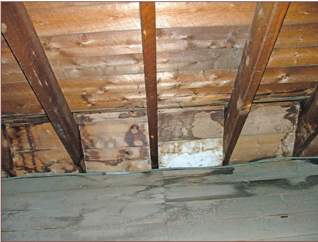
Figure 4 – Staining under roof deck and on floor.
