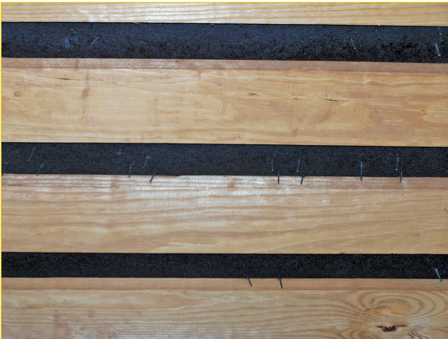
Photo 10 – Incorrect fastener application – nailing into air and missing the sheathing boards. The holding power of these fasteners is nil.
