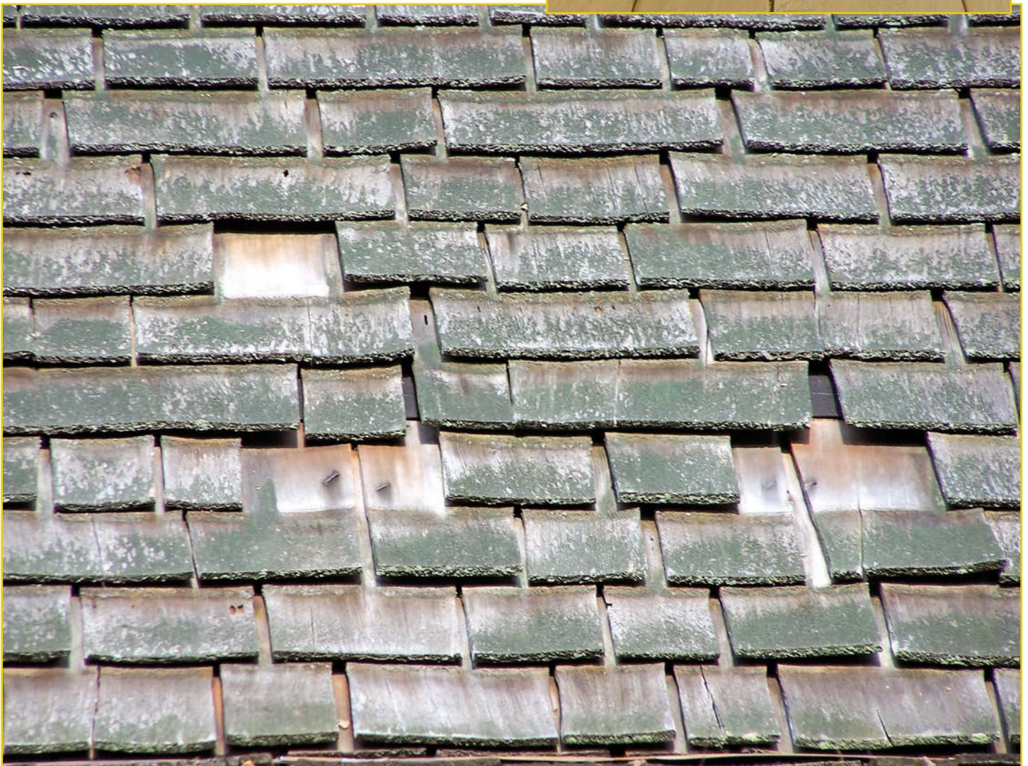
Photo 6 – Fastener issues causing roof failure.
