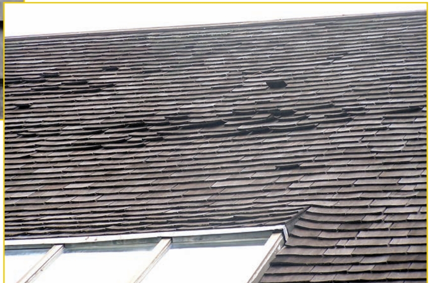
Photo 5 – Example of product lifting and curling due to installation of nonpermeable membrane across entire deck.
