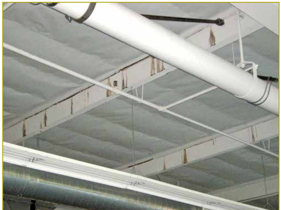
Figure 3 – Stains on the sides of beams in an office/warehouse building in California.
