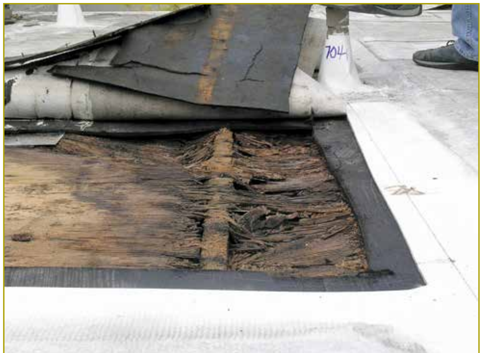
Figure 1 – Severely deteriorated plywood a few years after replacing an old cap-sheet BUR with a white single-ply roof.
