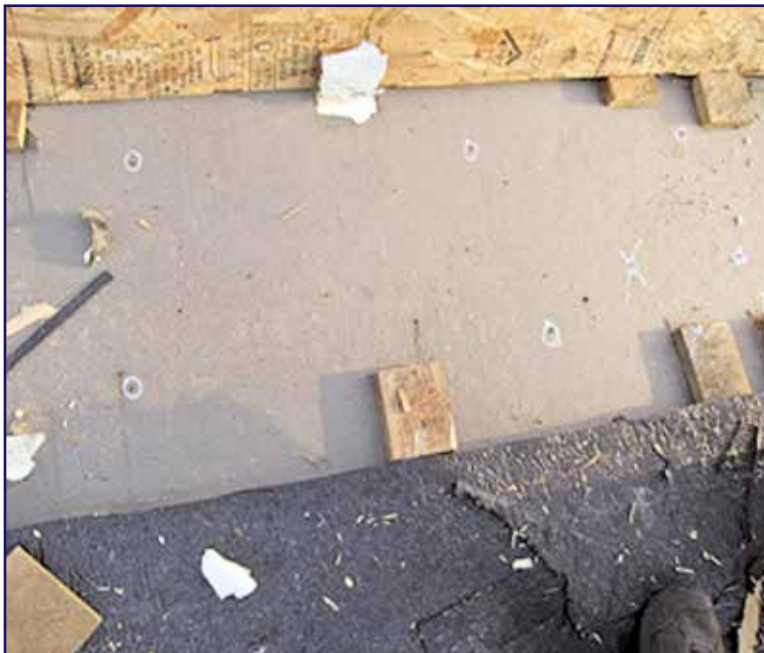
Figure 1 – Vented nailbase with sheathing cut out.
