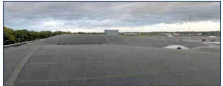
Figure 3 – Uplifted EPDM at compromised area.
