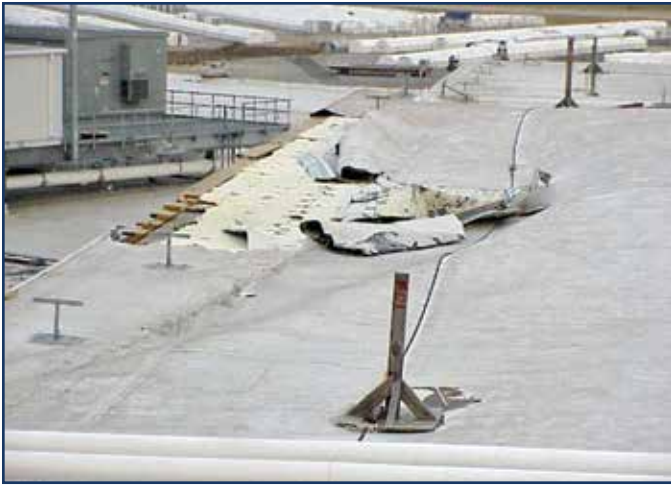
Figure 2 – Uplift damage to adhered PVC roof assembly.
