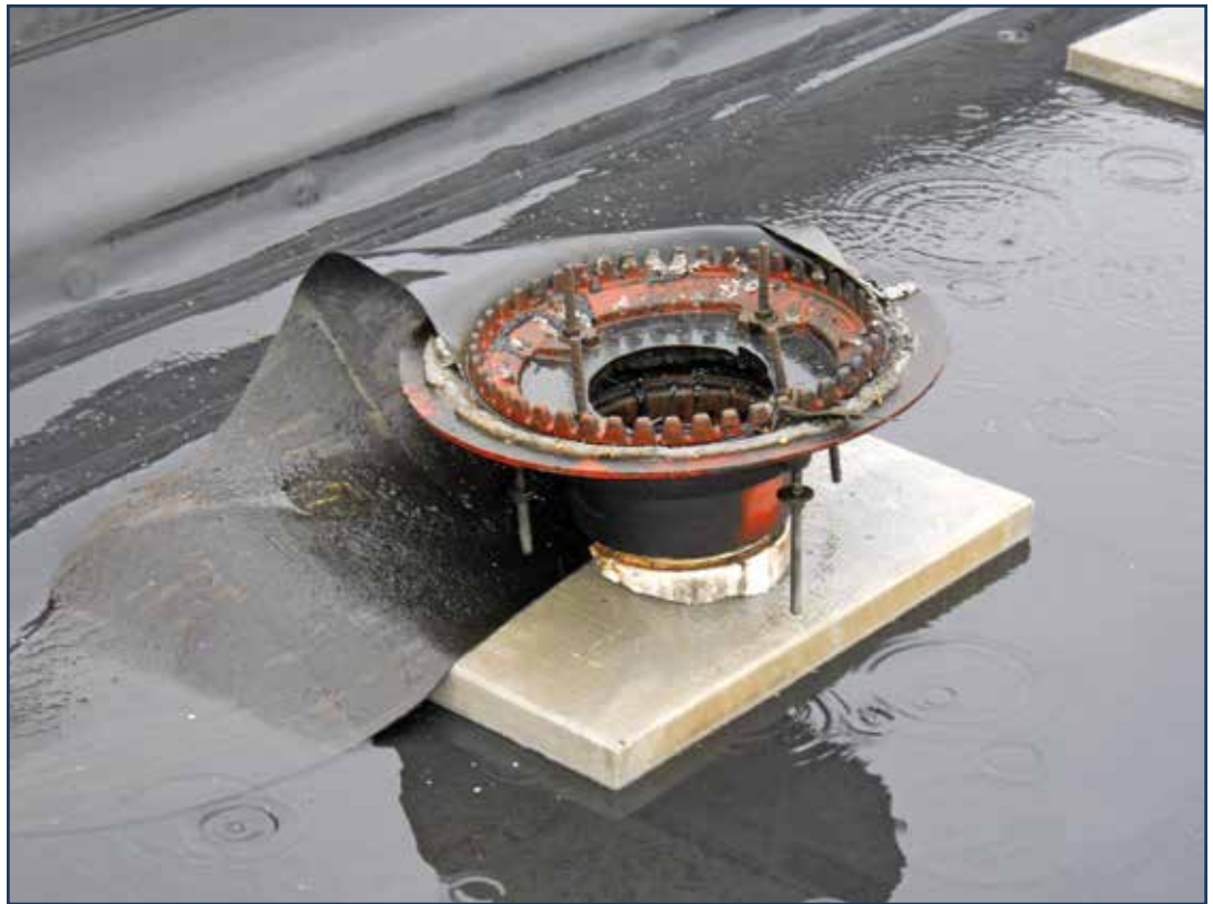
Figure 5 – Dislodged roof drain on uplifted EPDM area.
