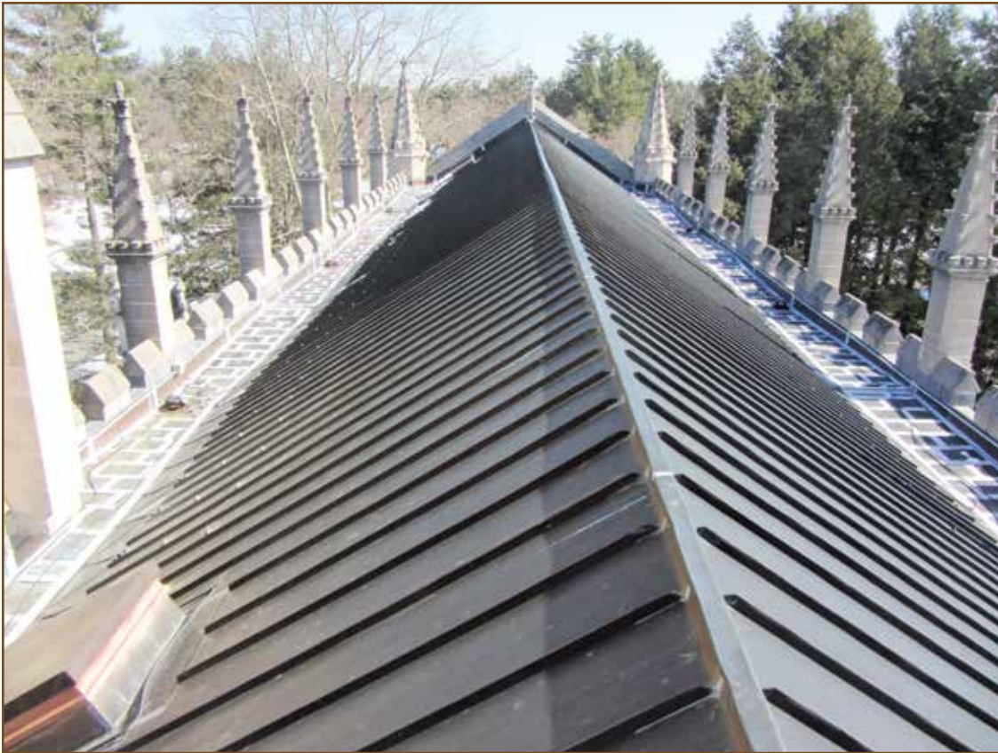
Photo 6 – Nave roof (note temporary gusset repairs).
