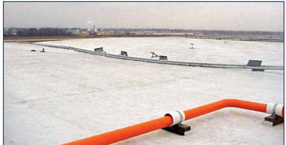
Figure 4 – Uplifted PVC roof at compromised area.
