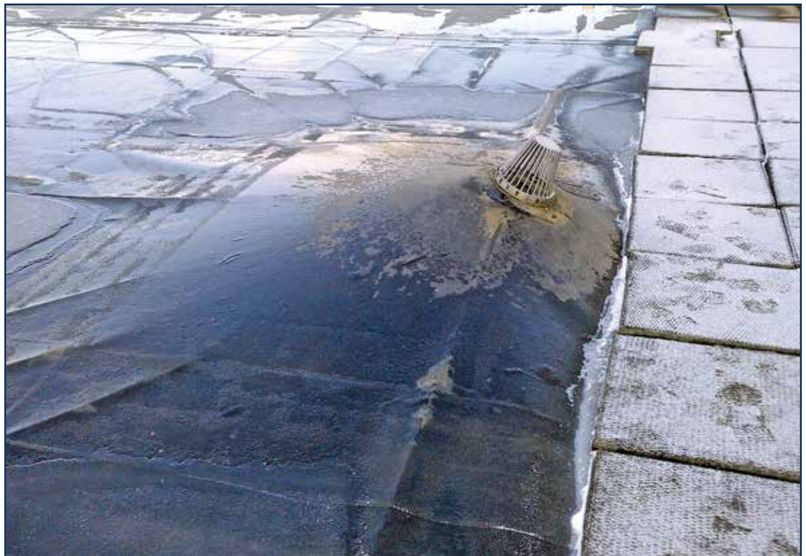
Figure 1 – The roof drain and cast-iron leader were dislodged by the uplift pressure on this roof system.
