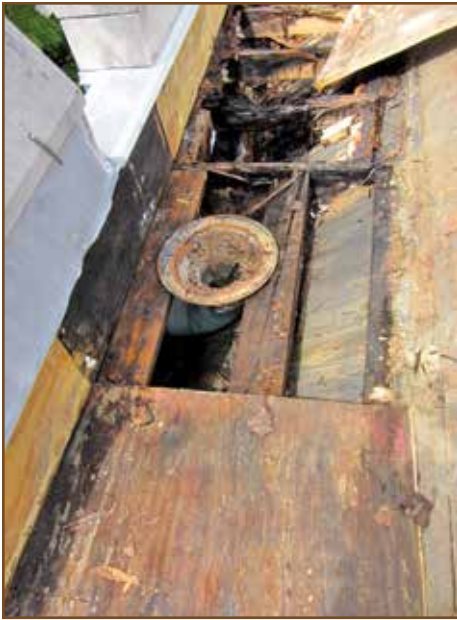
Photo 4 – 2000 gusset installation in 2011, with deteriorated framing from solder seam failure and condensation.
