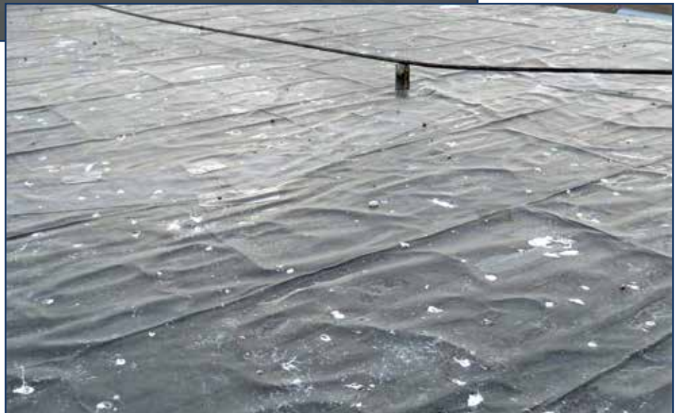
Figure 7 – Disbonded EPDM membrane with iso facer adhered to underside, pulled free of the foam core.
