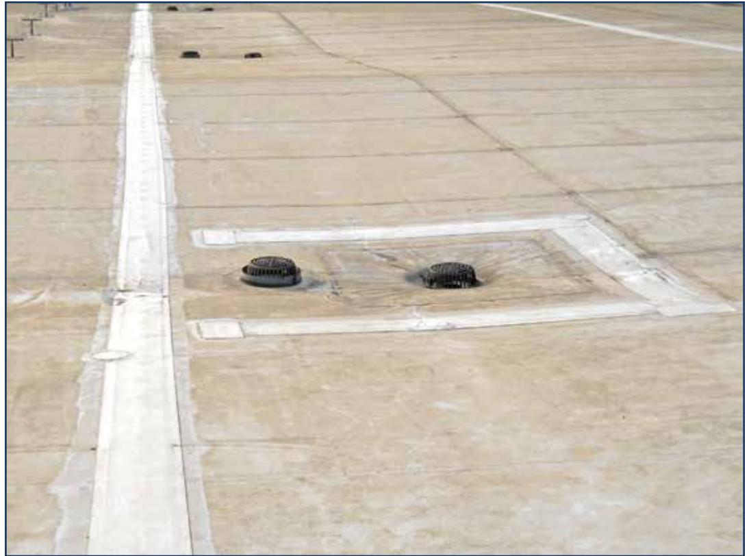
Figure 10 – Battens around roof drain on uplifted area.
