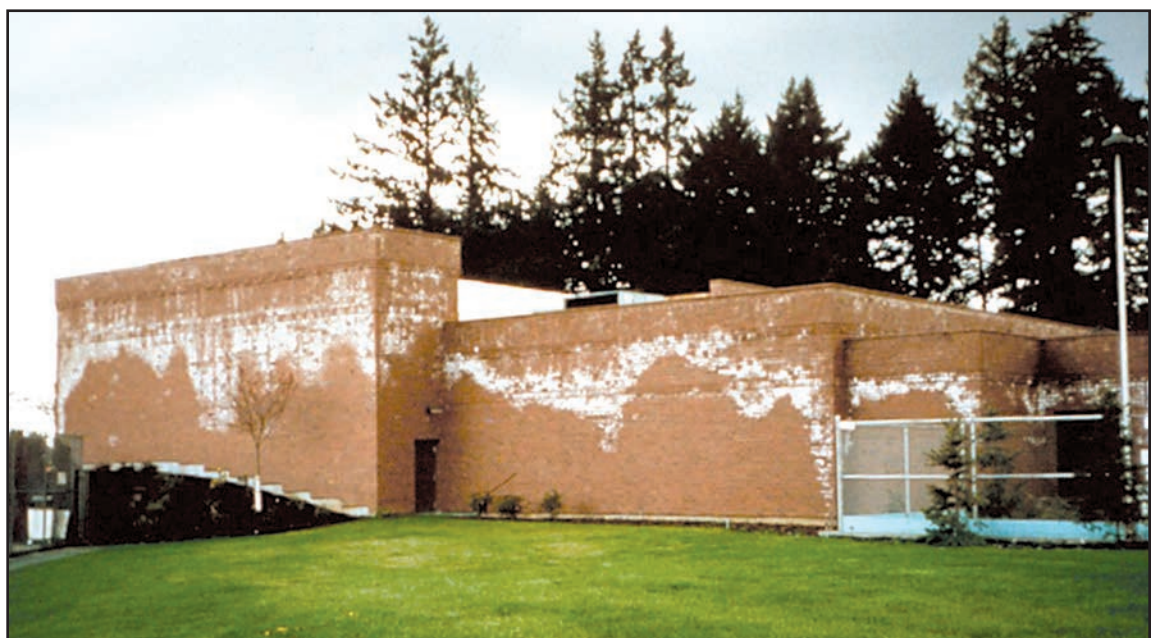
Figure 9: Efflorescence from rainwater penetration can quickly mar a beautiful new masonry façade. (Photo courtesy of Prosoco.)
