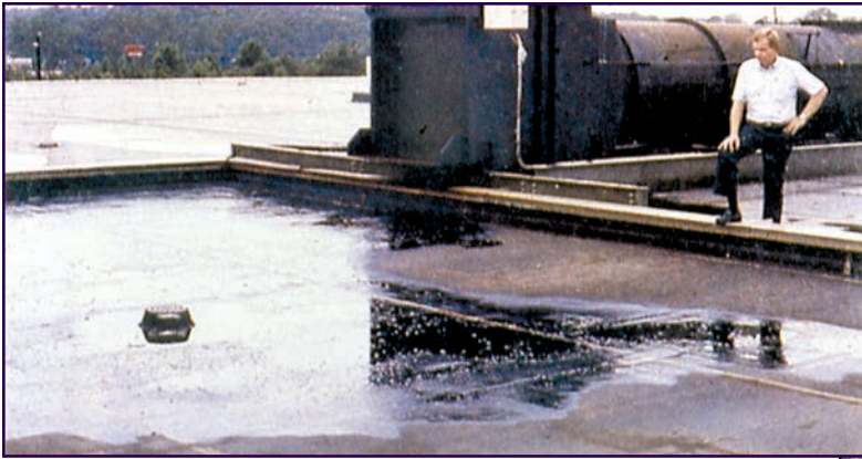
Figure 23: Polyepichlorohydrin rubber was used in this roof bay in order to resist oil contamination.
