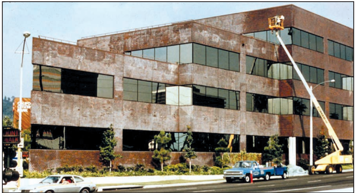
Figure 8: Workers remove sealer blush from a Southern California office building. Sealer blush results from using film-forming sealers on masonry. As water tries to evaporate out of the masonry, it is blocked by the film former. Eventually, the escaping water vapor breaks the sealer bond in spots. Where the sealer has debonded, more water from rain or other sources soaks in, leading to further debonding and more widespread sealer blush. The condition, as shown here, is correctable only by removing the failed coating, which can be expensive. (Photo courtesy of Prosoco.)
