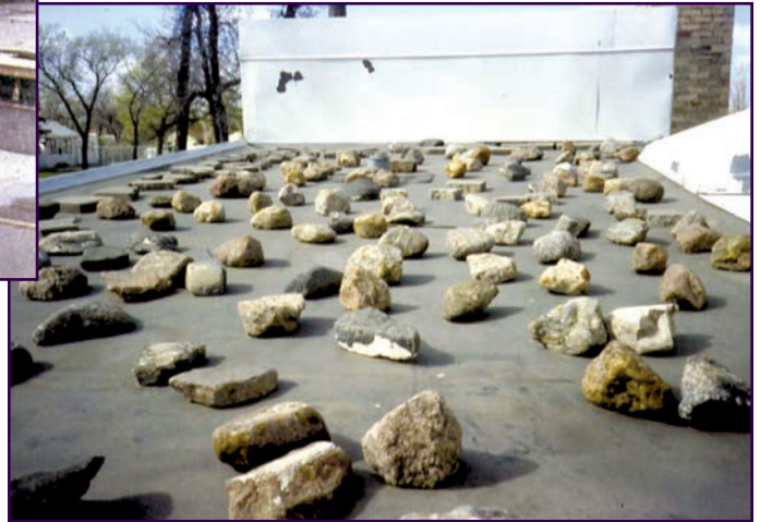
Figure 24: King-sized ballast on this roof!
