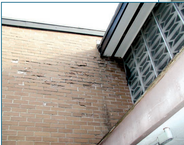
Figure 6: Faulty flashing leads to moisture accumulation and permanent freeze/thaw damage at roof interface.
