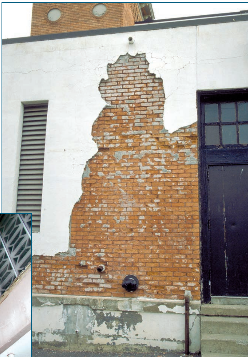
Figure 7: Freeze/thaw brick and parge coating failure.
