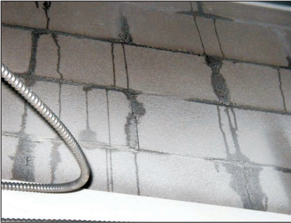
Figure 10: Single-wythe CMU: Interior view of integrally waterproofed CMU block and mortar. The head joints were not properly consolidated and did not prevent the passage of water during high wind events.
