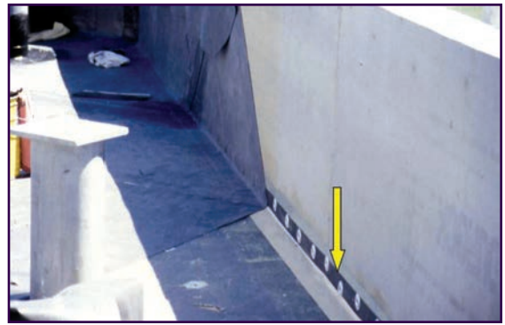
Figure 19: Edge restraint strips have reduced the tendency towards shrinkage and tenting of single-ply membranes.
