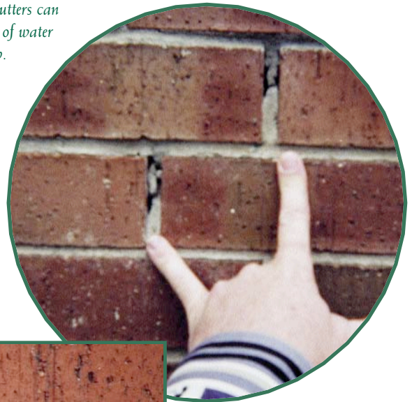
Above: Figure 3—Improperly filled mortar joints will admit significant amounts of water.
