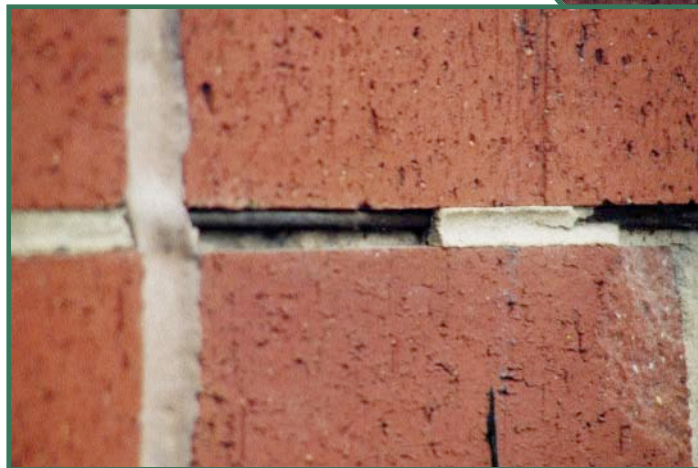
Left: Figure 4—Wire reinforcing within mortar joints is sometimes arranged too close to the outside face. This causes the thin mortar cover to break away, resulting in still more avenues for water entry.
