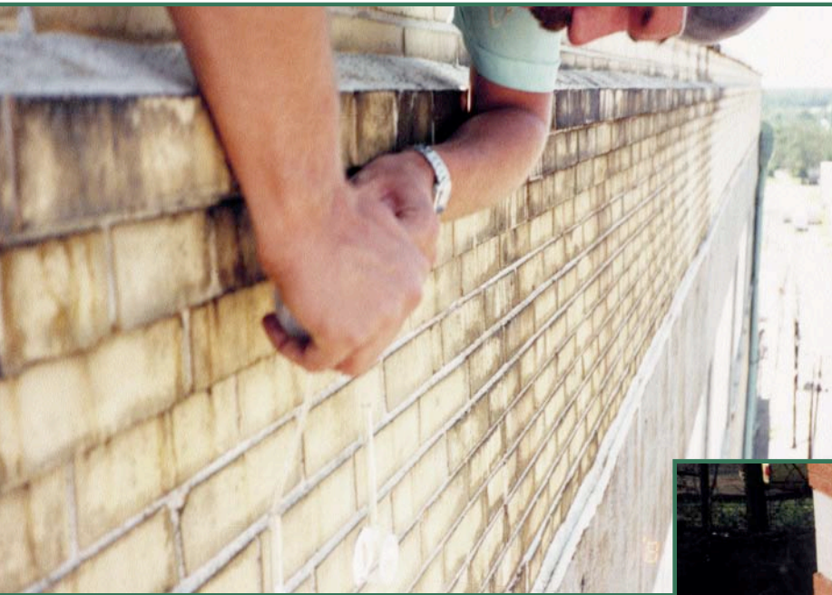
Figure 5—One method for determining the rate of water absorption into brick masonry construction is the RILEM tube test. Unfortunately, the test results are often misunderstood or misapplied. While quite valid for evaluating water-repellent treatments, the test is often meaningless for evaluating a chronically leaking wall.
