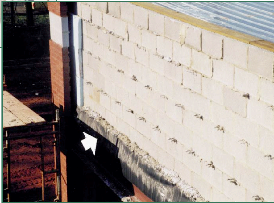
Figure 6—Cavities clogged with mortar are not functional avenues for water removal.
