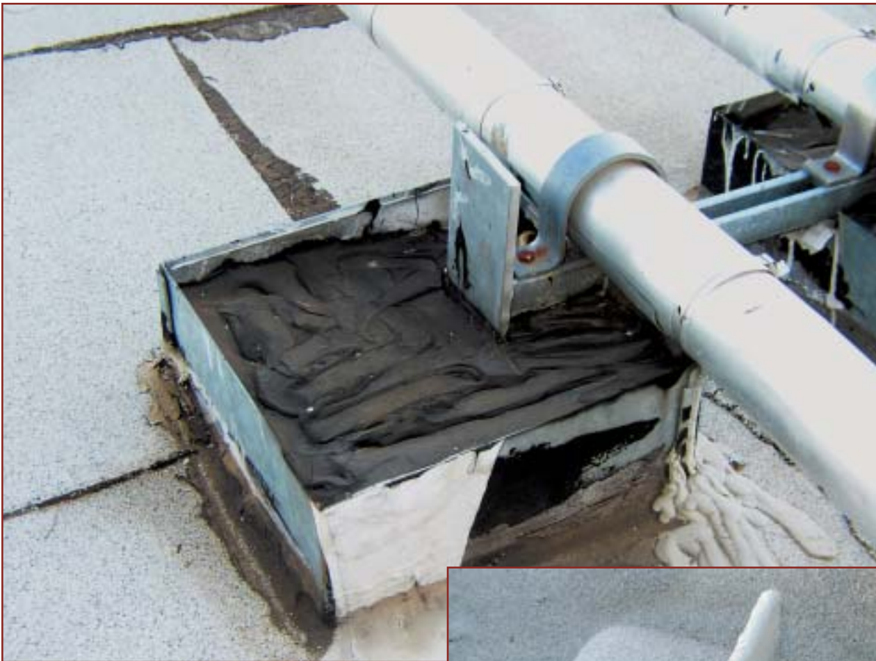
Old pitch pan with dried asphalt mastic.
