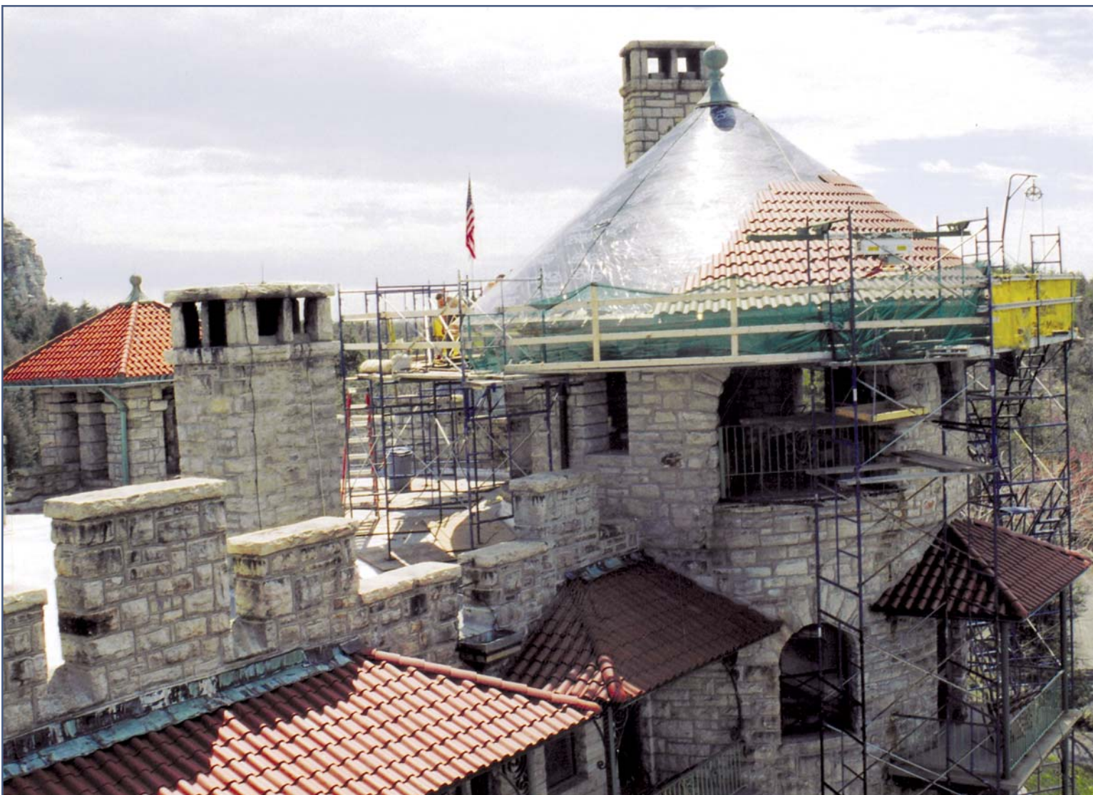
Photo 3 – Process of replacing original Ludowici Celadon clay Spanish tile (initially installed at the turn of the 20th century) with new tile by the same manufacturer on an historic hotel in upstate New York (the original tile came from Celadon's plant in Alfred, NY). Photo by Robert L. Fulmer.
