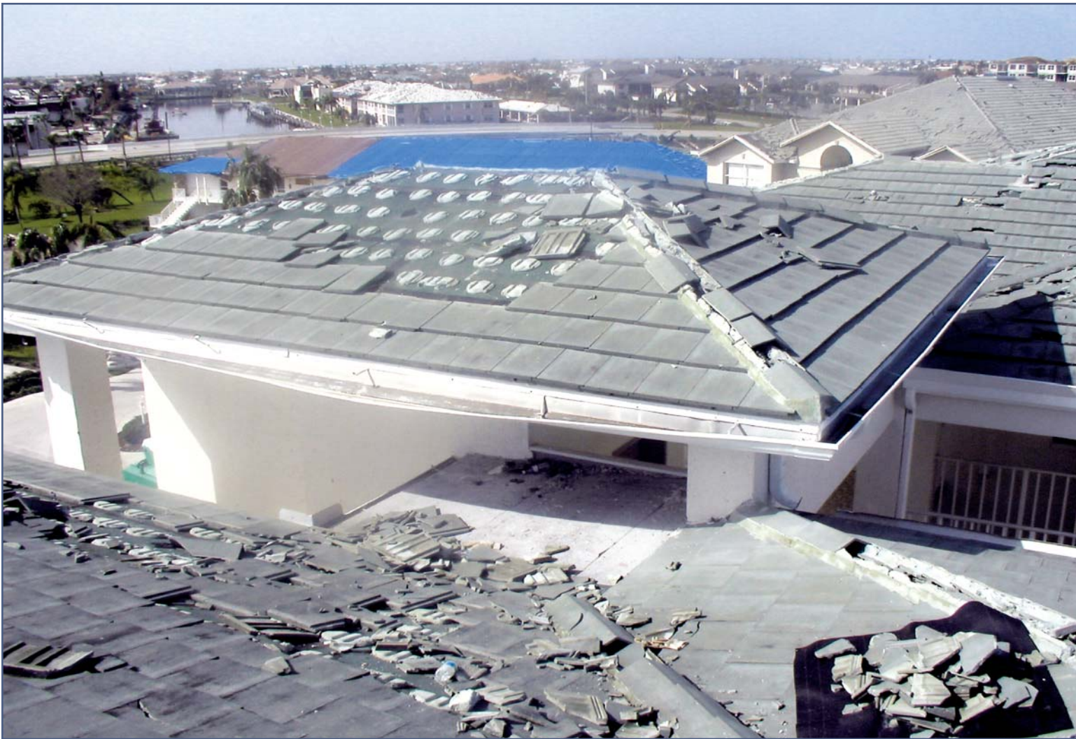
Photo 5 – Example of a ridge tile failure in a concrete tile roof system. Photo courtesy of Warren French.
