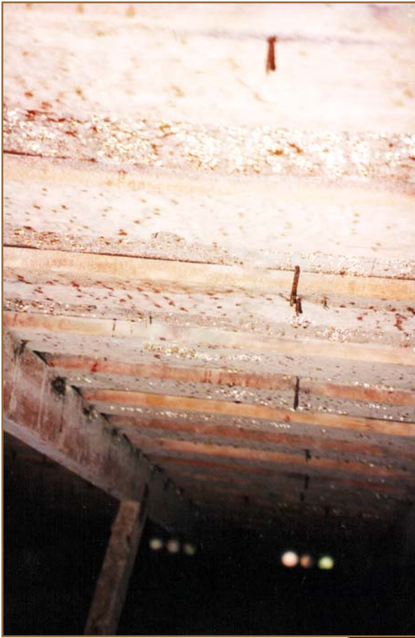
Photos 3 (left) and 4 (below) – Literally thousands of water droplets form on the underside of a plywood and spaced sheathing roof deck despite conventional attic eave vents on a project where a self-adhered membrane underlayment was installed as part of a roof replacement project.
