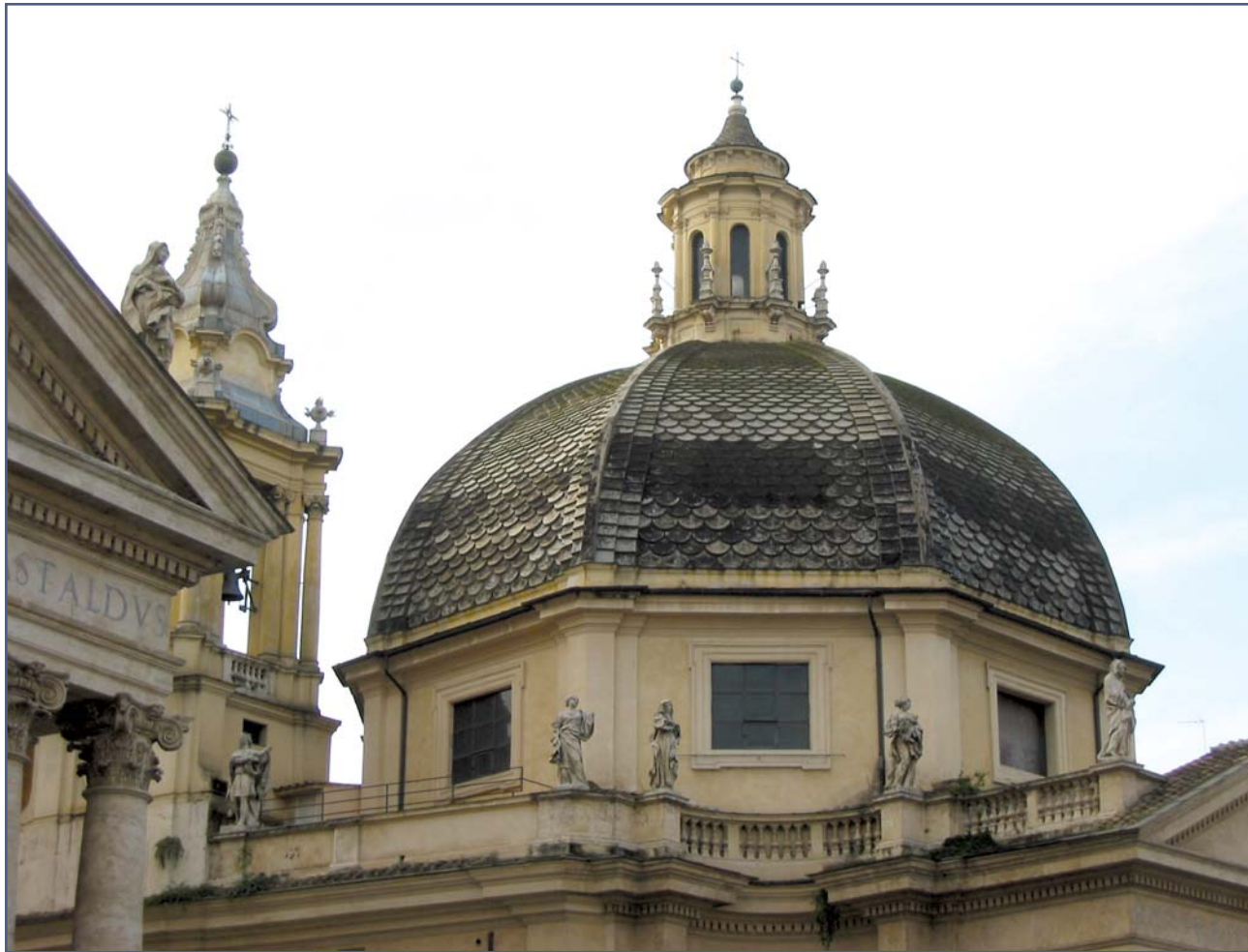
Photo 1 – Flat clay tile on a dome at the Pantheon, Rome, Italy. Photo by Robert L. Fulmer.
