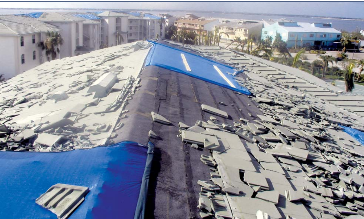
Photo 6 – Upper concrete tile roof exhibiting partial failure of the “foam-set” system, possibly due to an improper foam mix. Lower roof exhibiting damage from flying debris. Photo courtesy of Warren French.
