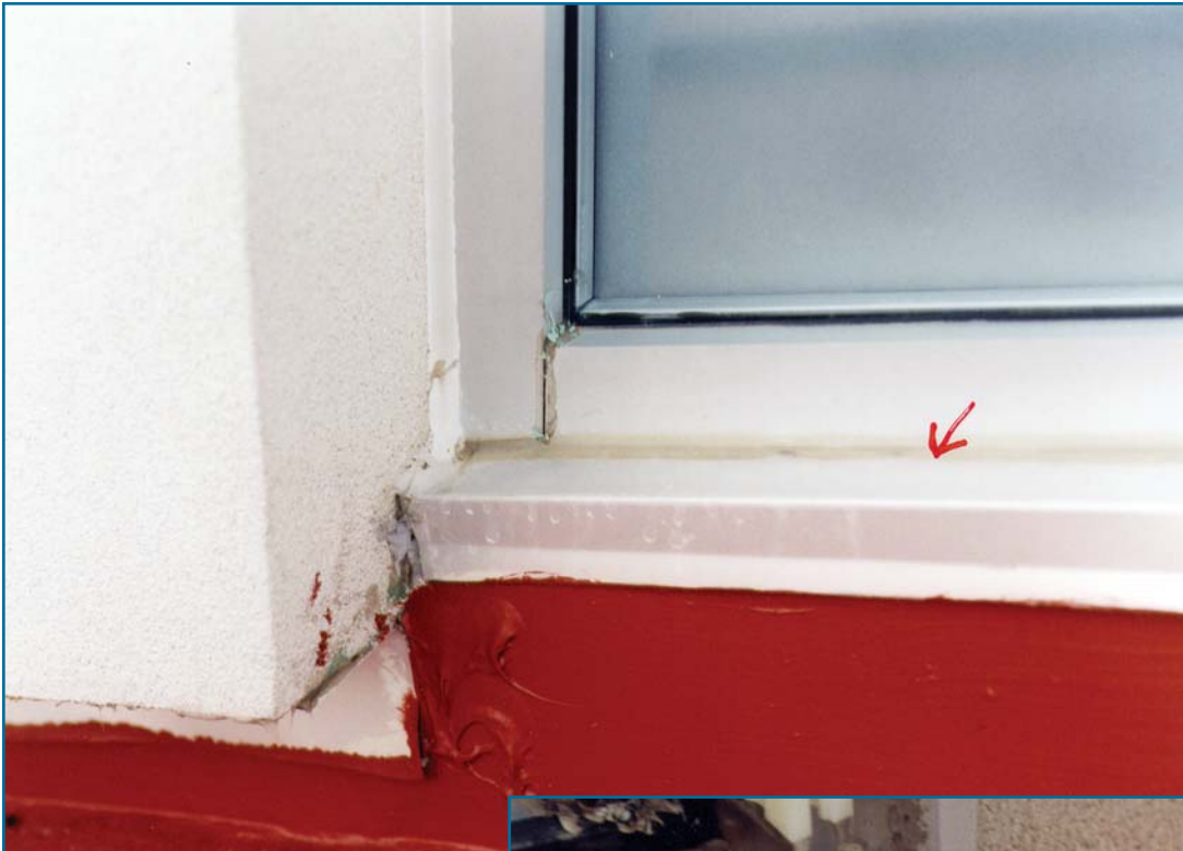
Figure 5: In a misguided attempt to solve the window leakage problem, the general contractor applied sealant (noted by arrow) at the drainage slot between the sill flashing and sill face cap.
