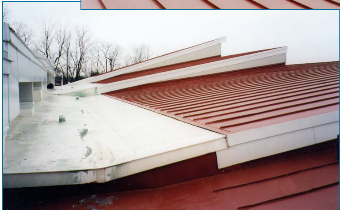
Figure 4: View of the TPO membrane in the valley area. Water falling from the TPO membrane eroded the paint on the terne below.
