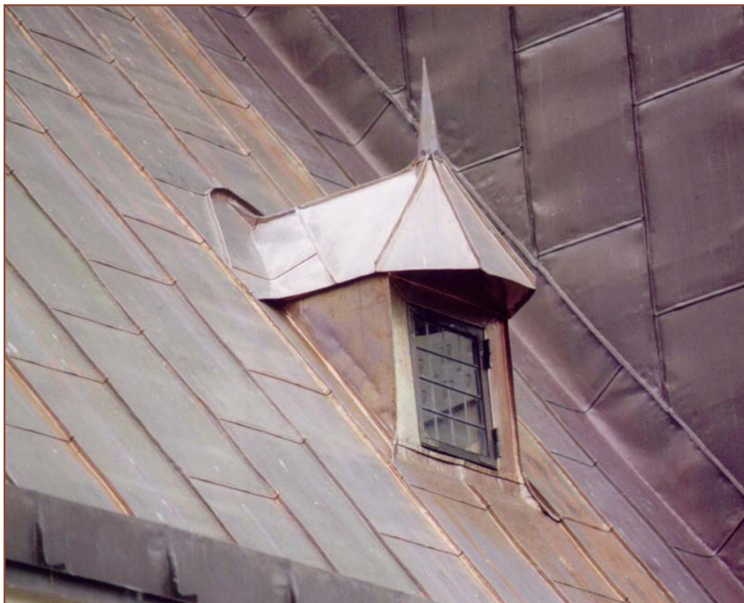
Greater detail and weather integrity can be accomplished with soft crafted metals as shown on the Kronborg Castle in Denmark.
