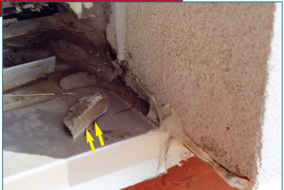
Figure 6: View of the down-slope end of the sill flashing after removal of the face caps and glazing. The only provision preventing water running down the sill from entering the building was a fillet-profile sealant joint between the sill flashing and EIFS. The double arrows show a piece of the sealant joint. The sealant was not well adhered to the EIFS or sill flashing. Water was able to flow past the sealant, where it had an unobstructed path into the building.
