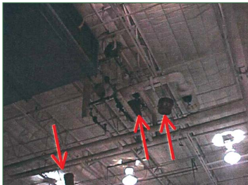
Photo 4: Buckets suspended from roof framing.
