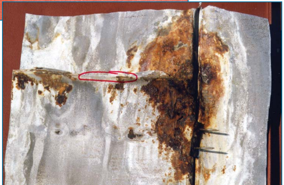
Right: Figure 9: View of the underside of the panel shown in Figure 8. The circle indicates the upper end of the down-slope panel. A panel clip with two nails occurs in the lower right portion of the photo.
