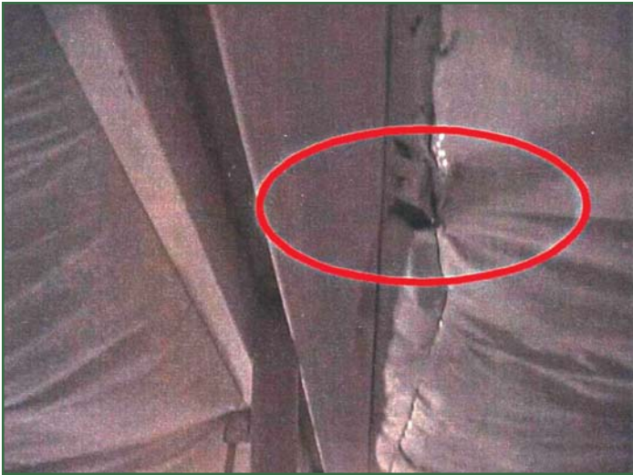
Photo 5: Insulation sidelap is “open” and not centered over framing member.
