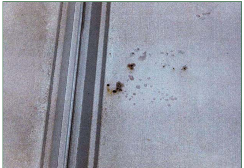
Photo 1: Moisture seeping through corrosion in roof panel.
