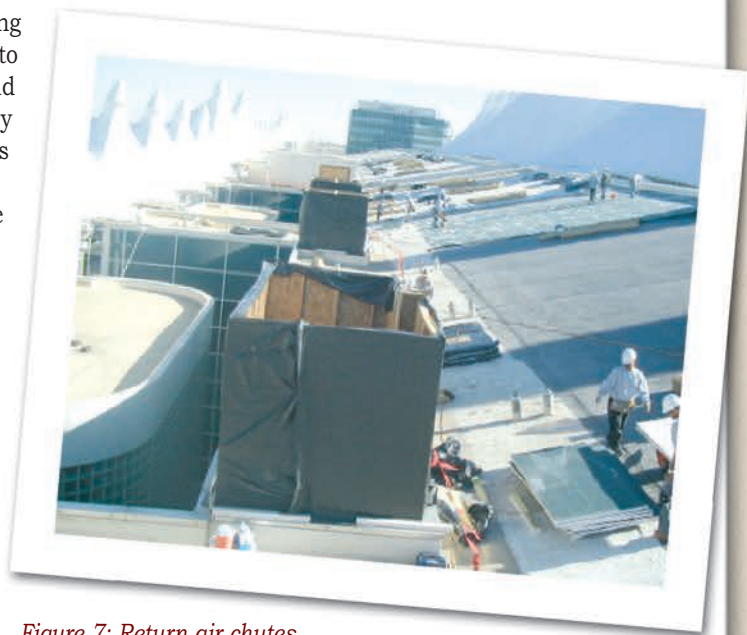
Figure 7: Return air chutes.
