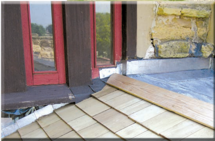
Photo 2: An addition to the old milk tower in the mid 1930s covered up an older terne-coated steel flat roof. The new ridge line resulted in an improvised surface flashing at a lower windowsill and the need for a saddle behind the tower wall.
