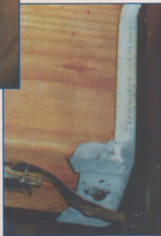
WHITE POWDER COVERING ENTIRE SUB-PURLIN HANGER
