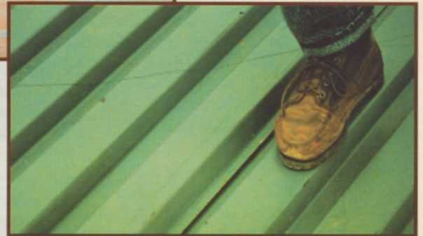
FIGURE 7. CONVENTIONAL STEEL DECKS DO NOT DEVELOP FULL DIAPHRAGM CAPABILITY UNTIL SIDE LAP STITCHING SCREWS ARE IN PLACE.
