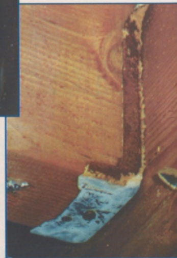
SURFACE RUST ON SIDE OF SUB-PURLIN HANGERS.
