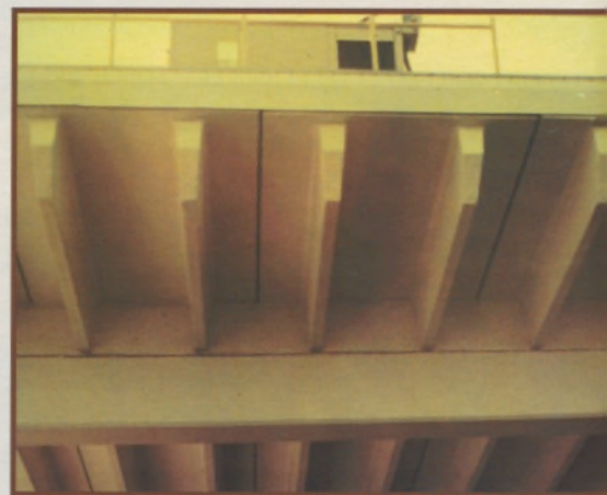
FIGURE 1. CONCRETE DECKS HAVE HIGH THERMAL INERTIA. WHEN COMPARED TO OTHER SUBSTRATES, ROOFTOP TEMPERATURE CHANGES ARE TRANSMITTED SLOWLY INTO THE BUILDING.
