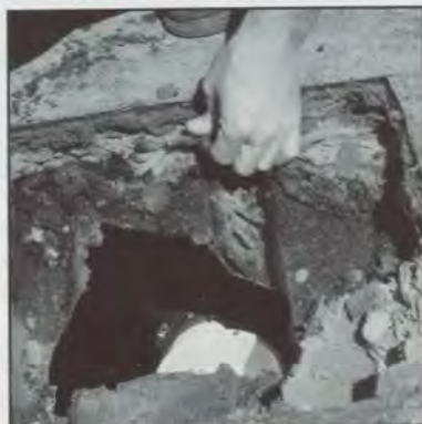
Drainage installation revealed the damp insulation of the old roof.
