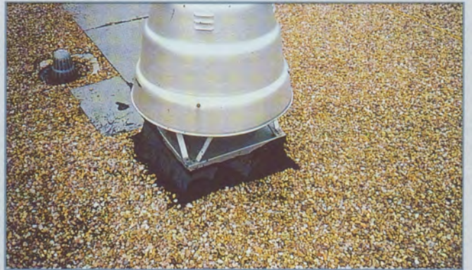
Rudd Hall. Missing fasteners in PRV.
