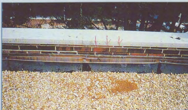
Masonry joint deterioration, typical.
