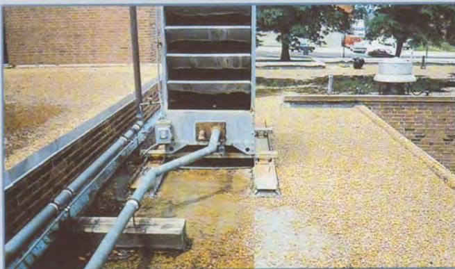
Roof Area A. Rust and corrosion on support and piping.
