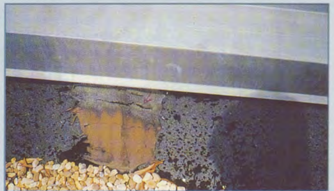
Bear Hall. Cracking roof cement base flashing joint cover.
