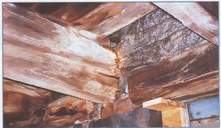
Water damaged wood joists.
