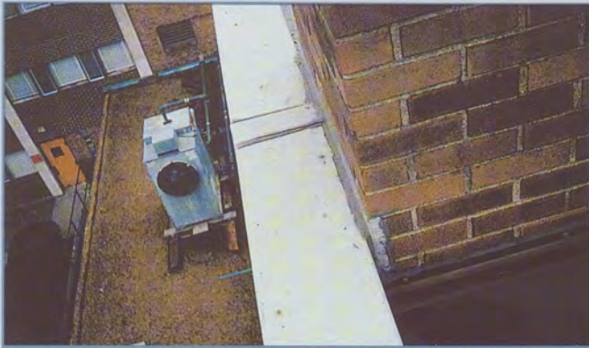
Rudd Hall. Deteriorated caulking behind chimney.
