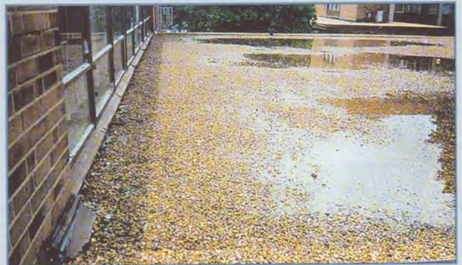
Roof Area B. Note loose flashing and low flashing profile below windows.
