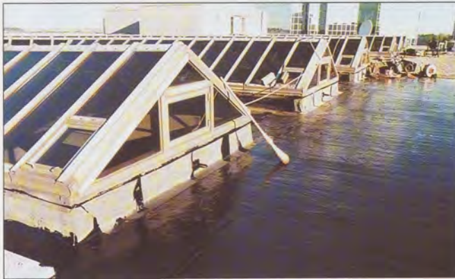
Fig. 9: The completed installation of the flat roof expansion joint. Note the vertical flashings.
