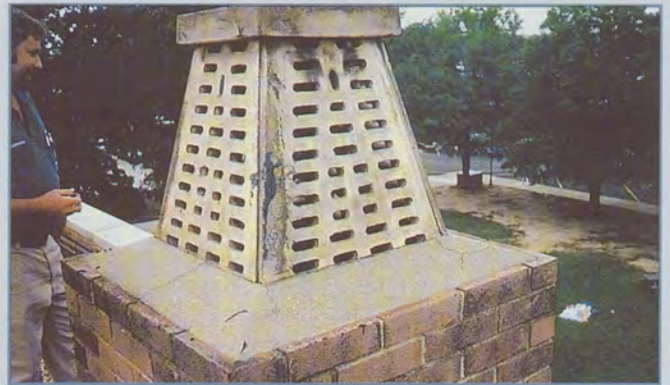
Rudd Hall. Poor waterproof seal on chimney.
