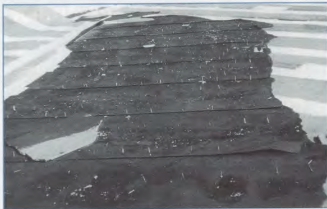
Improper base sheet application resulted in wind gusts less than 70 mph removing this section of roofing. Note the smooth shank roofing nails protruding up through the base sheet.
