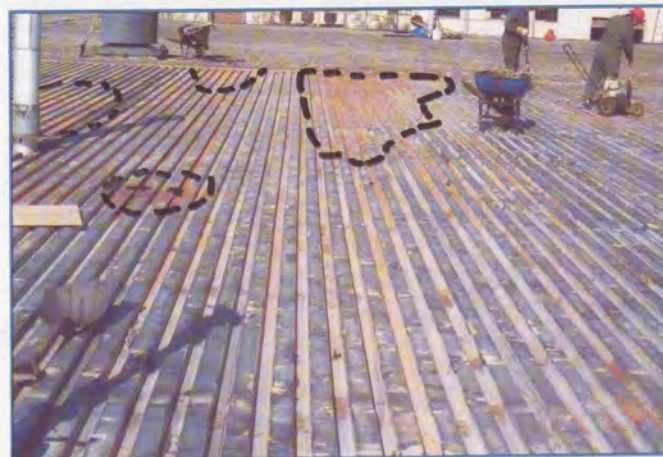
Photograph 5 - Case 2: BUR with fiberboard. Pattern of localized corrosion concentrated around leak locations shown by dotted lines.
