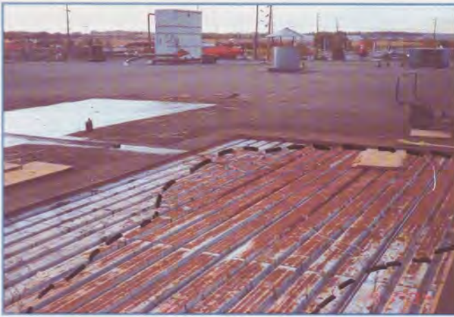
Photograph 7 - Case 3: BUR with Perlite. Corrosion concentrated around leak shown by dotted line. Corrosion on web (1), flange (2) and flute (3).
