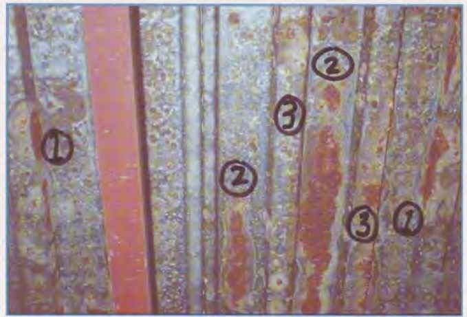
Photograph 8 - Case 4: BUR on concrete/steel deck composite. Corrosion on web (1), flange top (2) and bottom (3).
