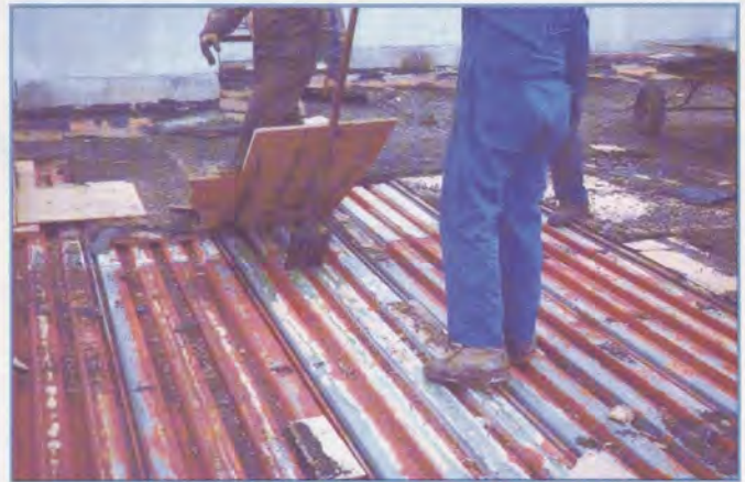
Photo 1 - Case 1: BUR with fiberboard. Corrosion on web, top flange and flute. Notice adhesive on back of insulation and no corrosion at adhesive location.
