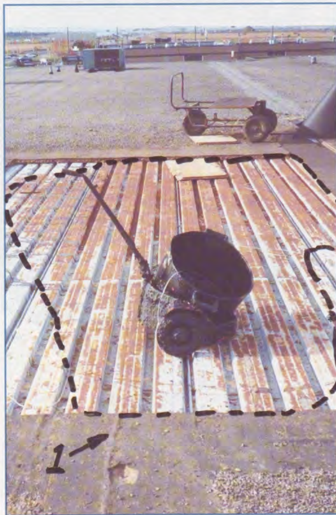
Photograph 6 - Case 3: BUR with Perlite. Pattern of localized corrosion concentrated around leak locations shown by dotted line. Notice ridge (1) in foreground in line with the center of maximum corrosion.
