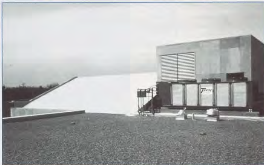
Typical stone-ballasted roof. These gain fire rating where some other roof types will not.
