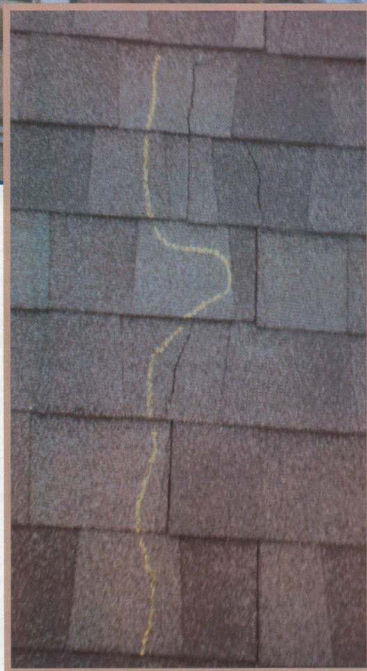
Shingles had split at many locations throughout the roof, both vertically and horizontally. Vertical splits are shown here.
