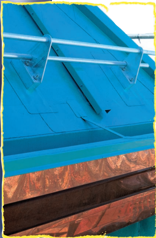
Simulated "pacific turquoise" copper roofing meets authentic copper soffit trim which, when aged, will match in patina green color.
