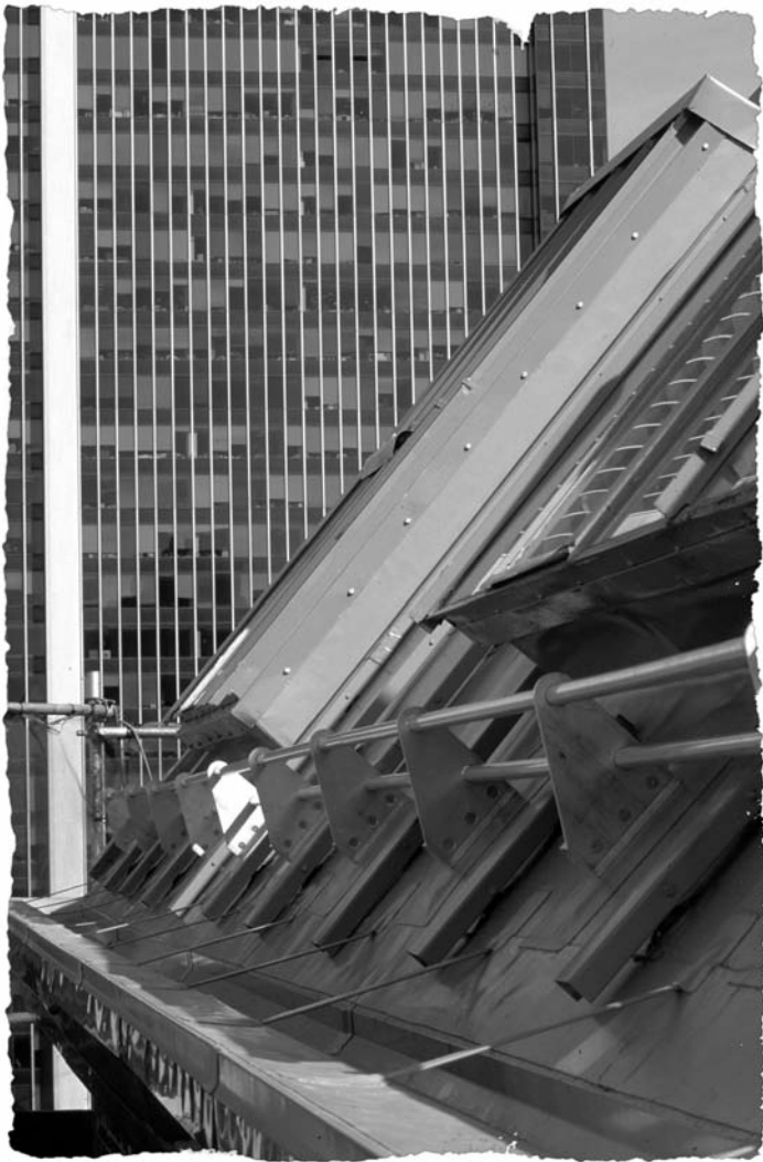
A detail of custom-manufactured skylights which perfectly match some 13 various-sized originals, as well as aluminum snowguard and flashing detail.
