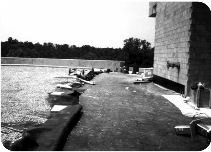
Above: Figure V—Termination of PMR system on Royal Center III.
