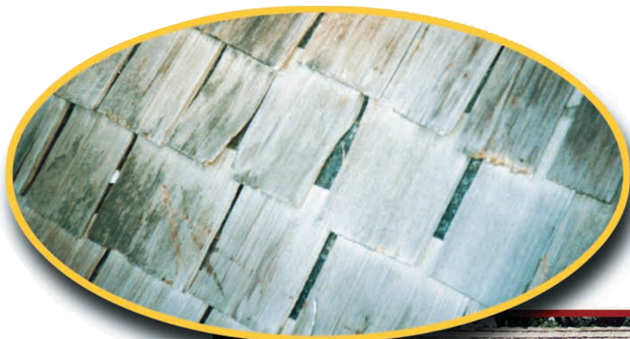
Figure 9—Felt interlayment should never show through in the finished array. "Rot-felting" may attract water upward to higher reaches of the installation. Moreover, the organic felt routinely used will not endure such exposure.
