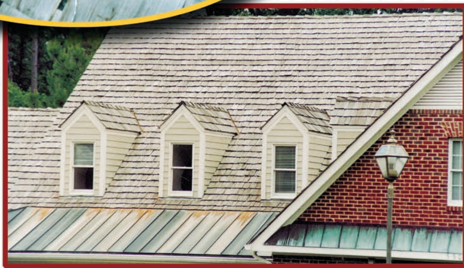
Figure 10—Runoff of certain chemical treatments may influence a copper roof covering. Note variation in patina. The permanency of all chemical treatments should be scrutinized.
