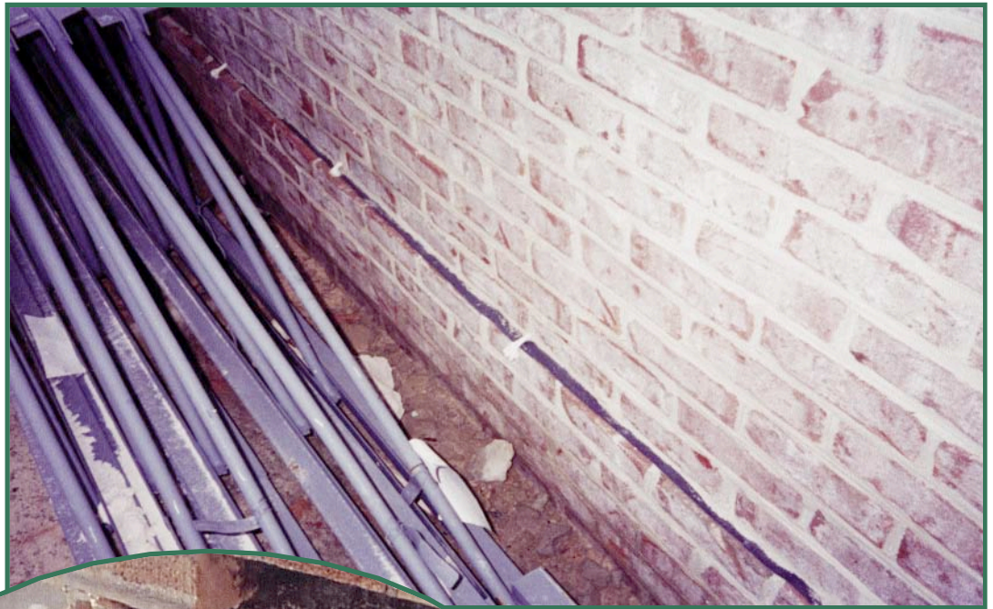
Above: Figure 8—Weep holes may be detailed with rope to attract water from the cavity of this wall.
