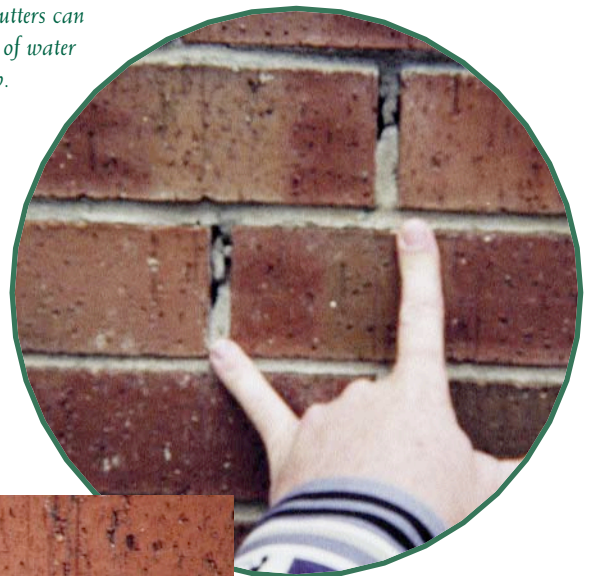
Above: Figure 3—Improperly filled mortar joints will admit significant amounts of water.
