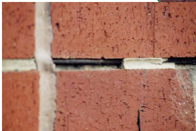
Figure 4—Wire reinforcing within mortar joints is sometimes arranged too close to the outside. This causes the thin mortar cover to break away, resulting in more avenues for water entry.
