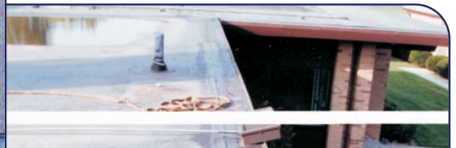
Left: Exhibit 4: View of pressurized seam using portable compressor. Water/soap solution used to locate leaks if present. Uniform profile of pressurized seam denotes correct adhesion area.
