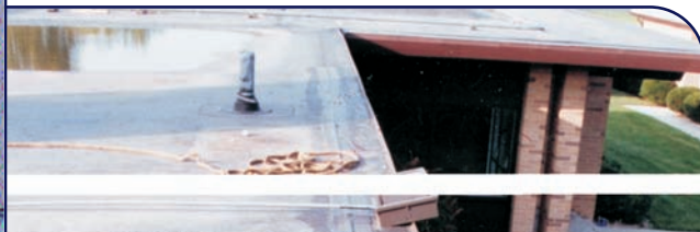
Left: Exhibit 4: View of pressurized seam using portable compressor. Water/soap solution used to locate leaks if present. Uniform profile of pressurized seam denotes correct adhesion area.
