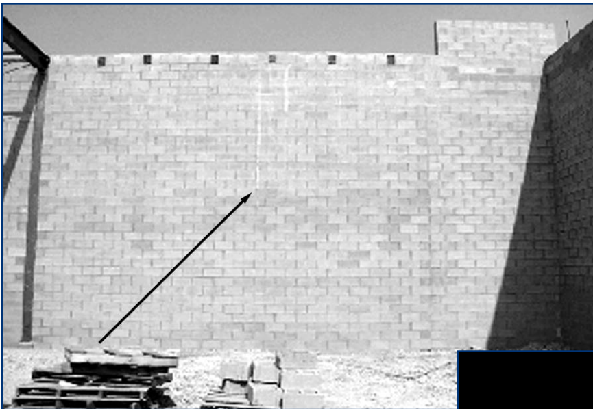
Figures 1 and 2) Photograph and thermograph of CMU wall with excess grout.
