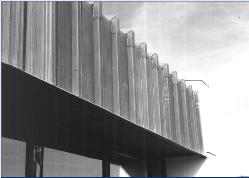
Above: Figure 5: A “fascia break” detail constitutes panel pinning because the vertical panel plane is cleated to the wall, inhibiting any movement along the slope of the roof at this interface.
