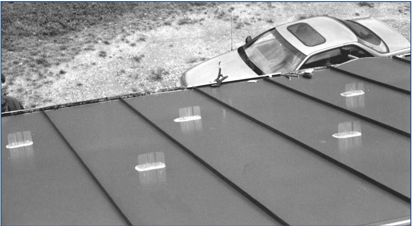
Figure 8: Snow guards which are mechanically fastened through metal panels and into the deck, constitute pinning of the panels at that location.
