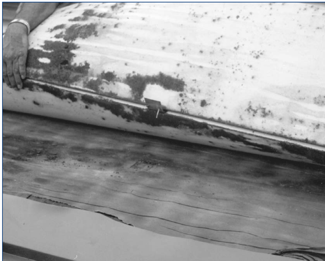
Figure 11: These panels are corroded through to perforation from the underside as a result of frequent moisture infiltration and felt saturation. They are two years old.
