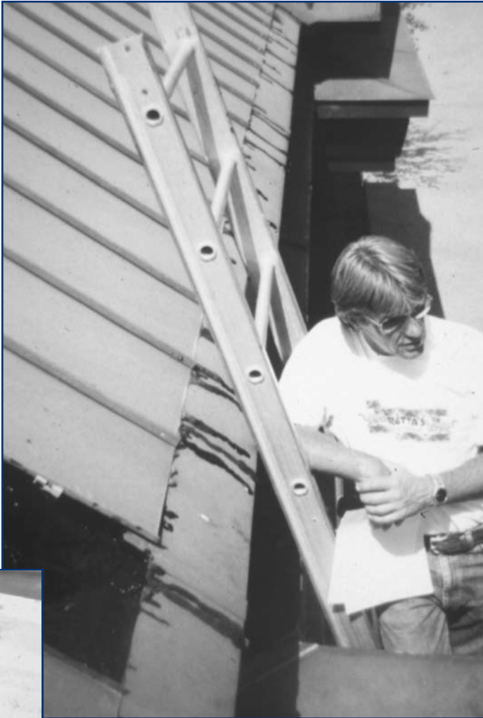
Above: Figure 12: Metal panels can get hot enough to exceed the softening point temperatures of some modified asphalt materials. This is especially true of dark colors and low gloss finishes.
