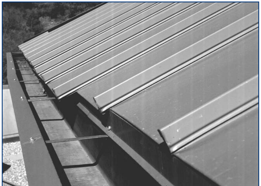
Figure 1: As long as the law of gravity remains on the books, panels that are not pinned will migrate down the slope of the roof.
