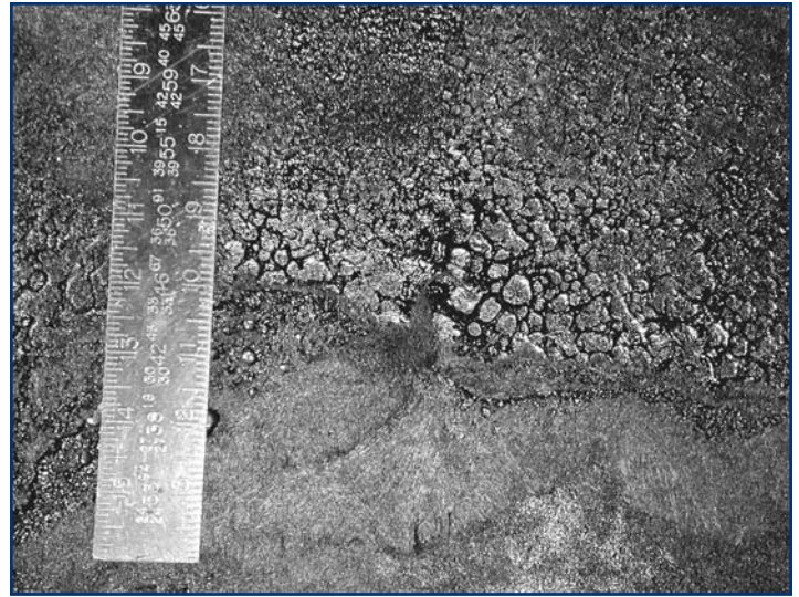
Photo 7—Observed blistering at facer-to-ply sheet interface.
