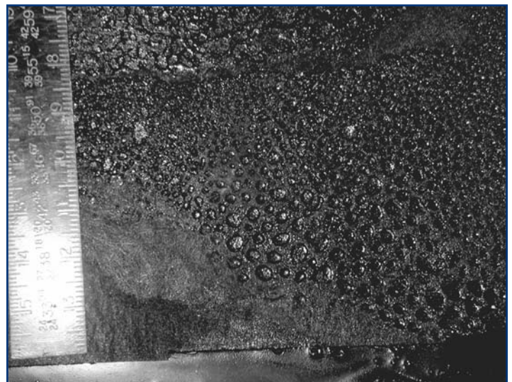
Photo 8—Observed blistering at ply-to-ply interface.
