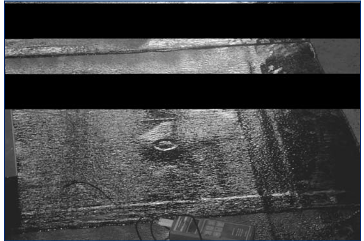
Photo 6—Blistering at stress plates, conventional torch application.
