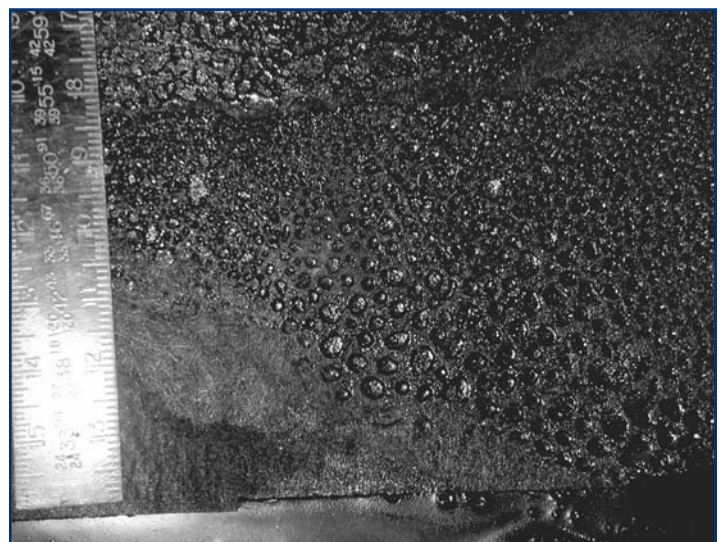
Photo 8—Observed blistering at ply-to-ply interface.
