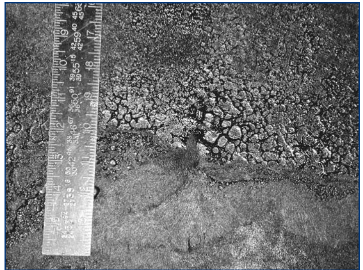
Photo 7—Observed blistering at facer-to-ply sheet interface.
