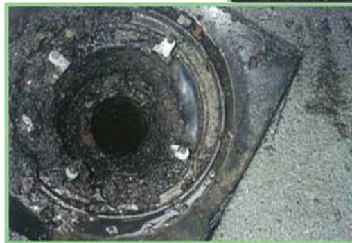
Original roof drain with dome removed. Note condition of the drain bowl.
