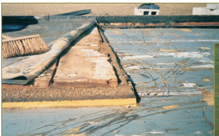
Photo 4—Uniform shrinkage of insulation used as a recover product.
