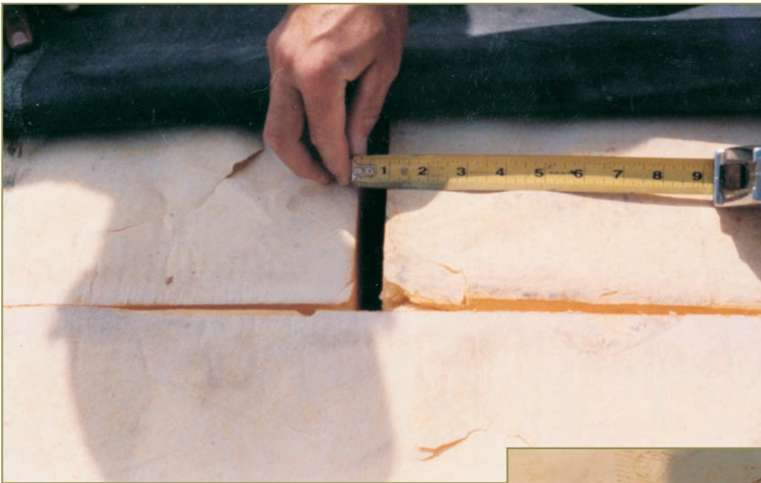
Photo 2—Careless installation of boards and the resulting gaps.
