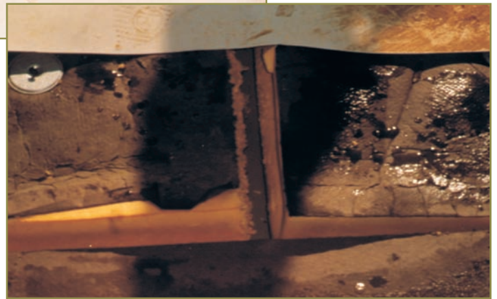
Photo 3 (below)—Uniform shrinkage of insulation boards. Water accumulation is from condensation on membrane underside.
