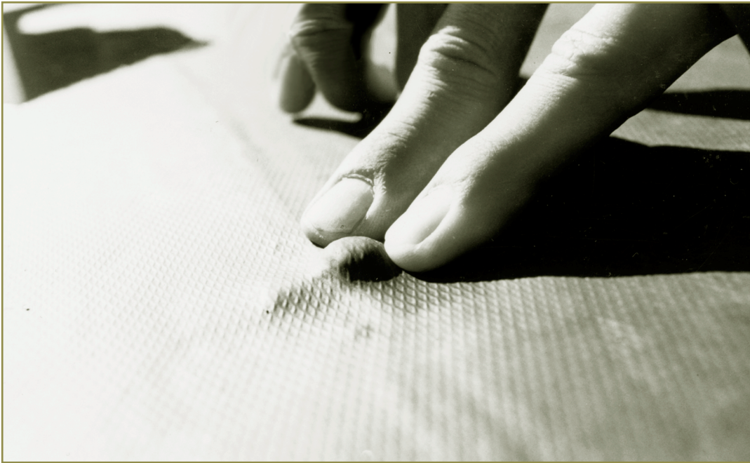
Photo 6—High (tenting) fastener, subject to puncture of a single ply membrane.
