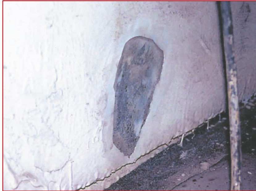
Figure 10 – Large blister at the base of a marine tank.
