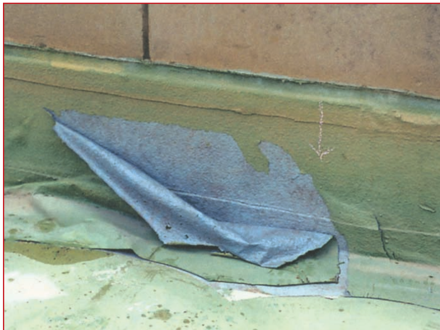
Figure 3 – Typical example of interlayer disbonding of the membrane between the green top coat and the gray base coat.
