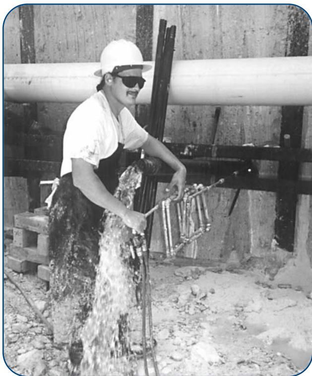
Figure 14: Water forces its way around casings for tie-back anchors and into a below sea-level excavation during construction of a Honolulu high-rise office tower. The injection contractor stemmed the flow with rags and oakum long enough to permit injection of fast-reacting chemicals around casings. Leaks were stopped and construction proceeded. (Photo by Structural Systems Inc.)
