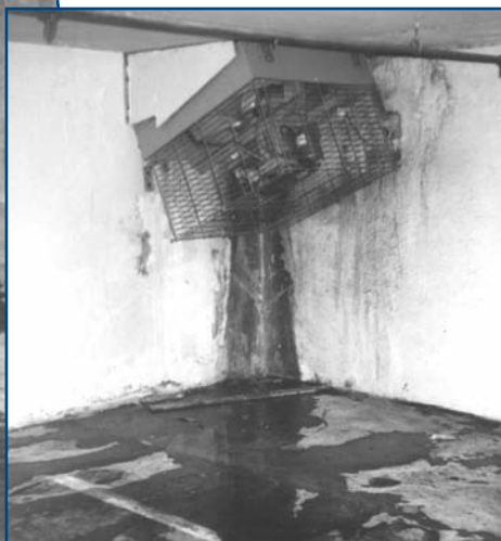
Figure 5: Above, a constant stream of water down this ventilation shaft and through two levels of parking resulted from waterproofing failure at cracks through foundation walls. (Photo by Phil Haisley.)
