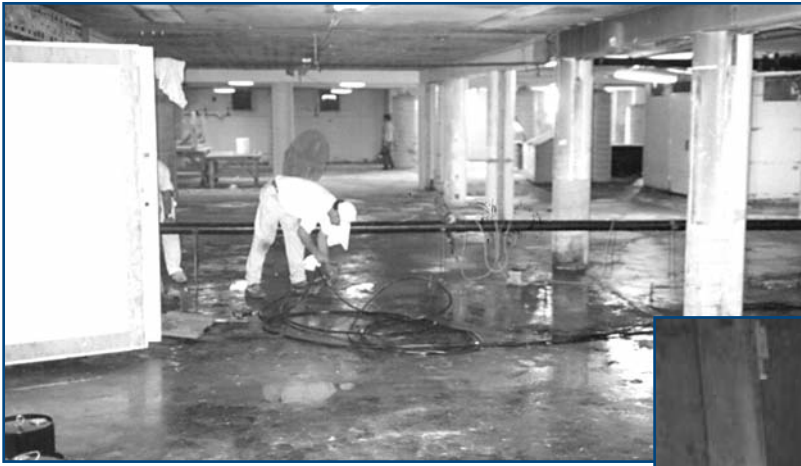
Figure 10: Standing water in the Waikiki basement above came and went with the tide, through slab cracks, foundation walls, broken floor rains, and sump pits. (Photo by Structural Systems Inc.)
