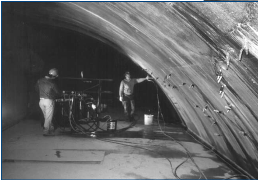
Figure 12: Waterproofing was "value-engineered" out of this highway tunnel project! Injection chemicals solved subsequent water intrusion problems at cracks through the concrete vault. (Photo by Structural Systems Inc.)
