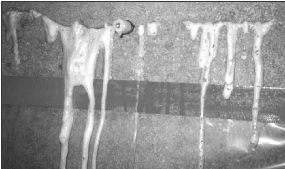
Figure 13: Surfaces of cracks are typically left unsealed for chemical injection. Ports are flushed with water to clean cracks and check communication between ports and are then injected until cracks are filled with chemical. Surface residues are easily cleaned after injection resins cure. (Photo by Structural Systems Inc.)
