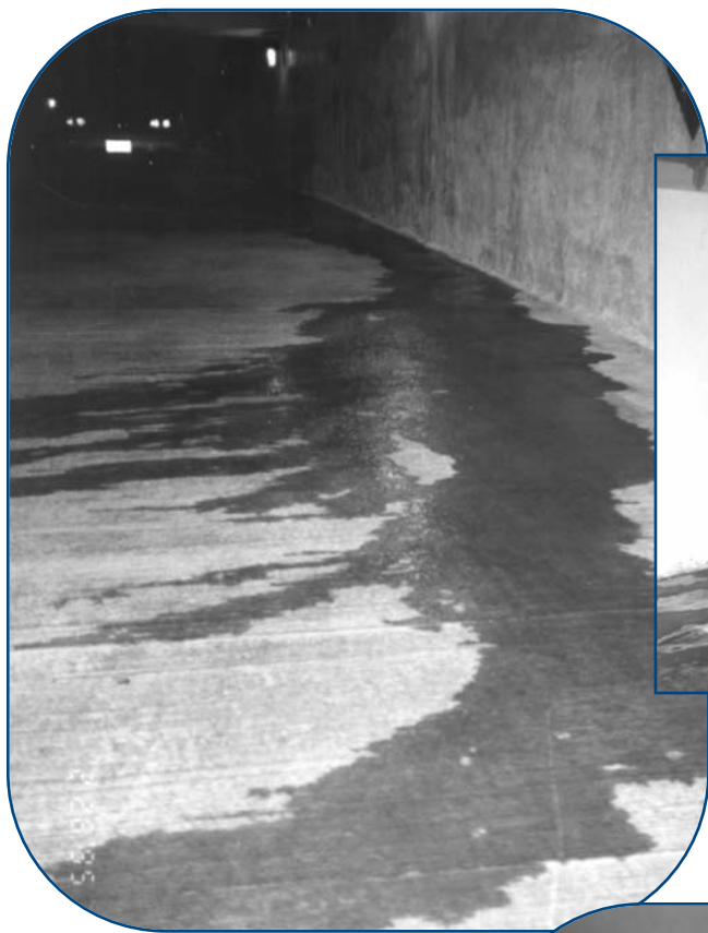
Figure 4: Above, hydrostatic pressure forced water through construction joints between the slab and foundation wall. This slab is approximately 15-20 feet below the water table. (Photo by Phil Haisley.)
