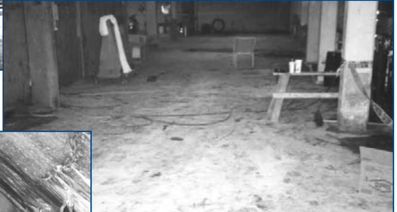
Figure 11: Above, the same basement slab shown in Figure 10 after a combination of gel and foam injection sealed slab cracks and created a soil barrier under the slab and around sump pits. (Photo by Structural Systems Inc)
