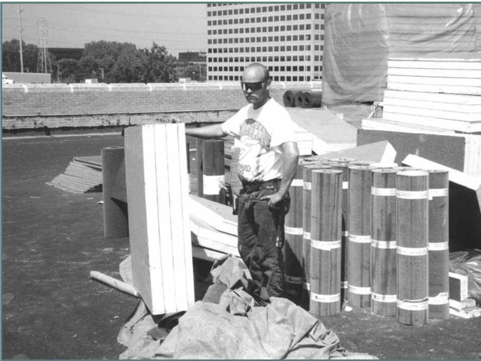
Photo 3. Tapered insulation with offset joints in sufficient thickness to provide substantial thermal value is an important consideration in the design of environmentally friendly roof systems. These sections of tapered insulation were prefabricated offsite, installed over a vapor/air retarder on two inches of polyisocyanurate, and overlain with a Perlite board. Meets Tenets 2, 7, 8, 9, 15, and 17.
