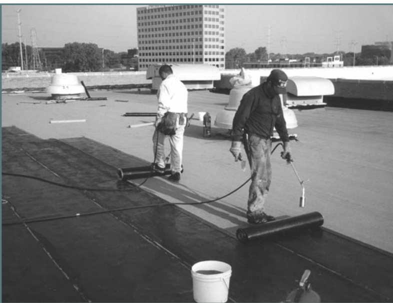
Photo 1. This roof system, composed of three modified layers on tapered insulation, was designed by the author and recognizes the value of a robust and durable roof. Taking the long view is the single most important concept in sustainable roofing. Meets Tenet 8, 9, 10, 13, 14, 16, and 18.
