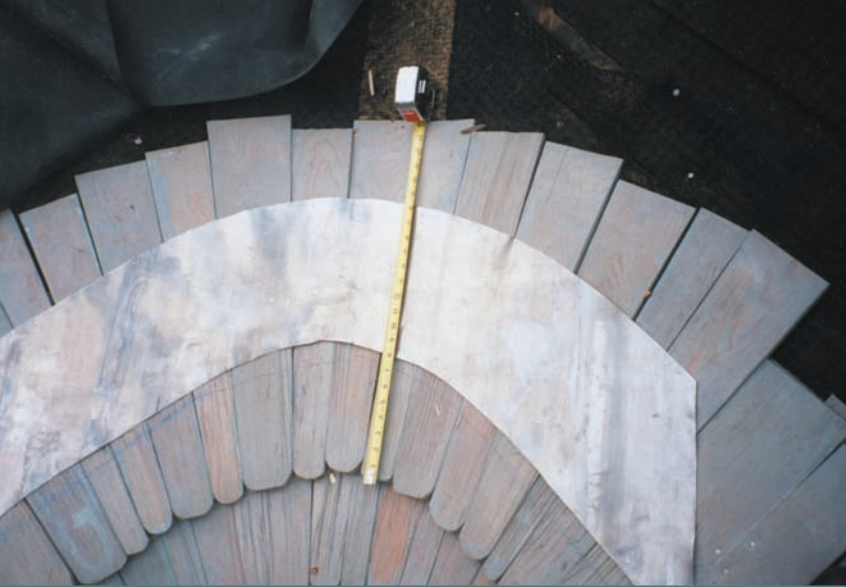
Photograph 4—Swept valley construction. Note the 24" valley shingles, which are tapered and have very narrow tips. Geometry of this construction does not permit the joints to be offset from one course to course below; therefore, the lead "step" flashing was installed. Also, note the adjacent 18" shingles. The longer shingles in the valley are necessary due to the increased exposure required within the sweep of the valley.
