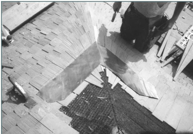
Photograph 7—Fanned hip construction. Note the 24" hip shingles, which are tapered and have very narrow tails. Geometry of this construction does not permit the joints to be offset from one course to course below, therefore, the lead "step" flashing was installed. Also, note the adjacent 18" shingles. The longer shingles at the hip are required due to the increasing distance as the shingles approach the hip in the wood deck.
