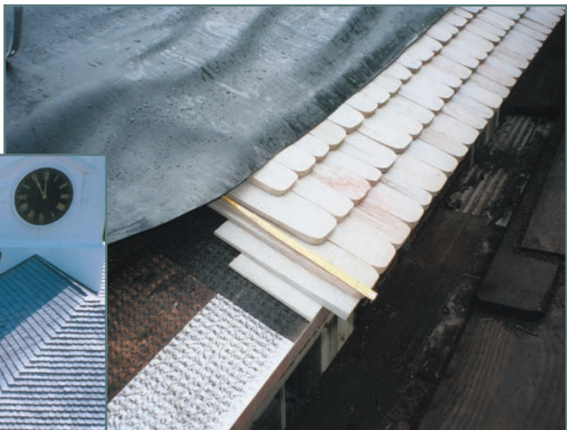
Photograph 3—Typical eave construction viewed from scaffolding during construction. Shows wood deck, edge metal, ice and water shield at eave only, Cedar Breather, two starter courses of wood shingles, and the new cypress shingles.
