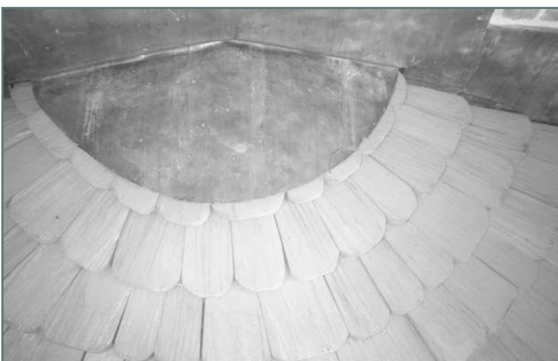
Photograph 13—Fanned shingle installation at apse roof. Note the lead cap at the peak of the apse shingles. Not visible is the lead interlayment under the course of wood shingles below the lead cap.
