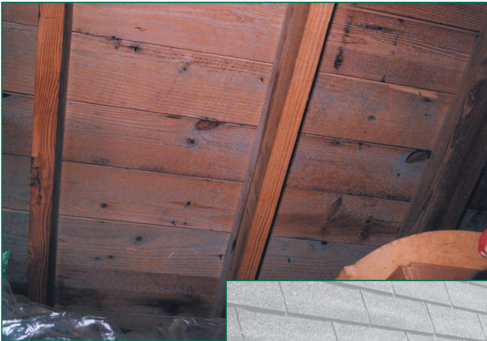
Figure 6—Mold/mildew in a humid southern climate. While attic insulation was properly held back at the edge and openings were present in the soffit cladding, the eaves carpentry was continuous along the entire perimeter. The mold/mildew colonies were fostered during a wintertime condensation scenario, drying to the powder during the hot season as shown.
