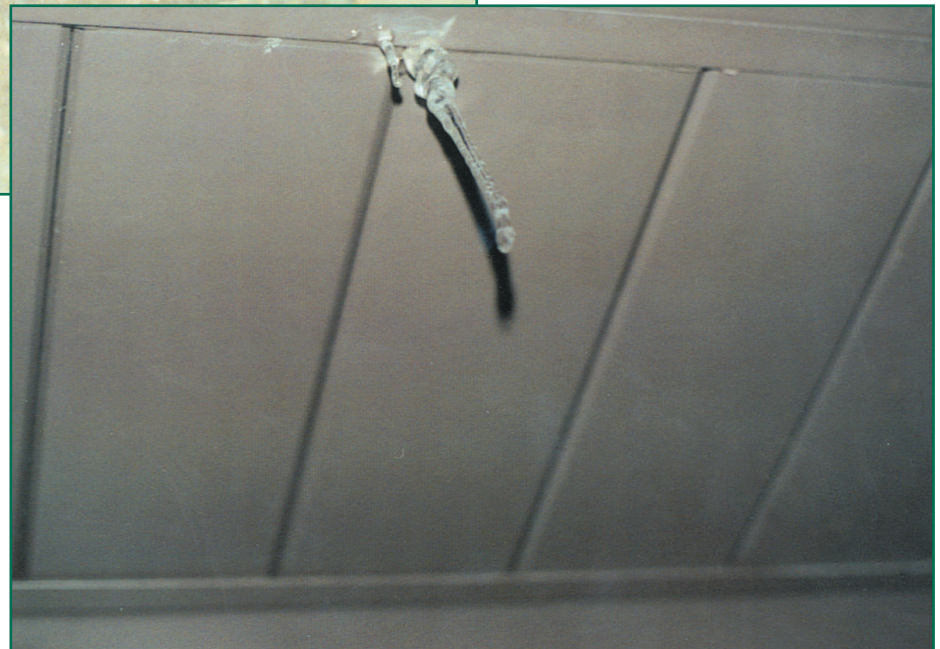
Figure 1A and 1B (below)—Ice damming on a roof where ice and water membrane was not provided.
