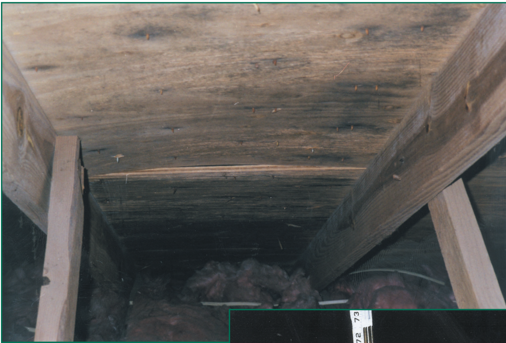
Figure 2—Moisture will accumulate in a wood deck long before water droplets are formed. Note the buckled plywood deck, mold formation, and soffit region blocked with glass fiber insulation
