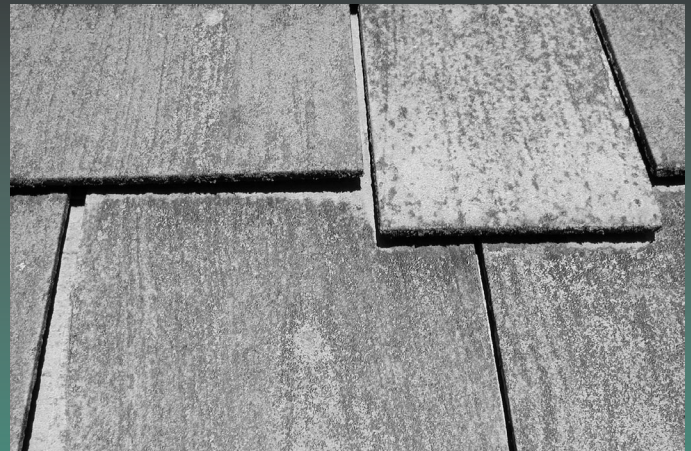
Photo 1 – Typical blackish algae growth observed throughout the project complex.
