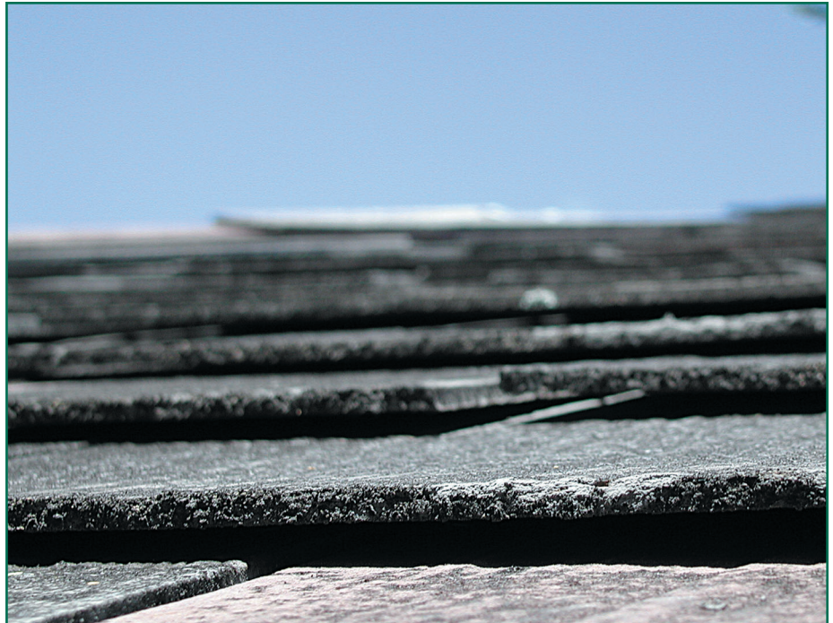
Photo 3 – Crumbling deterioration at leading edge
