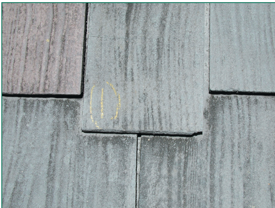
Photo 2 – Typical blackish algae growth observed throughout the project complex
