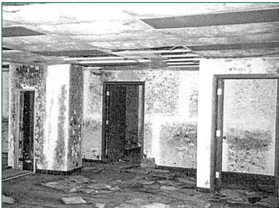
Mold permeates the ceiling, walls, and floor of this room. Can it be cleaned, and who is going to pay?
