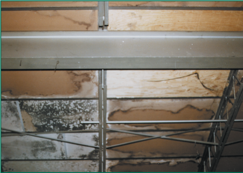
Figure 4: Formboards of a poured gypsum deck having been exposed to cycles of wetting. Repeated wetting in this manner will culture fungal growth. Concerns about indoor air quality can be traced to this condition, particularly in a return air plenum.
