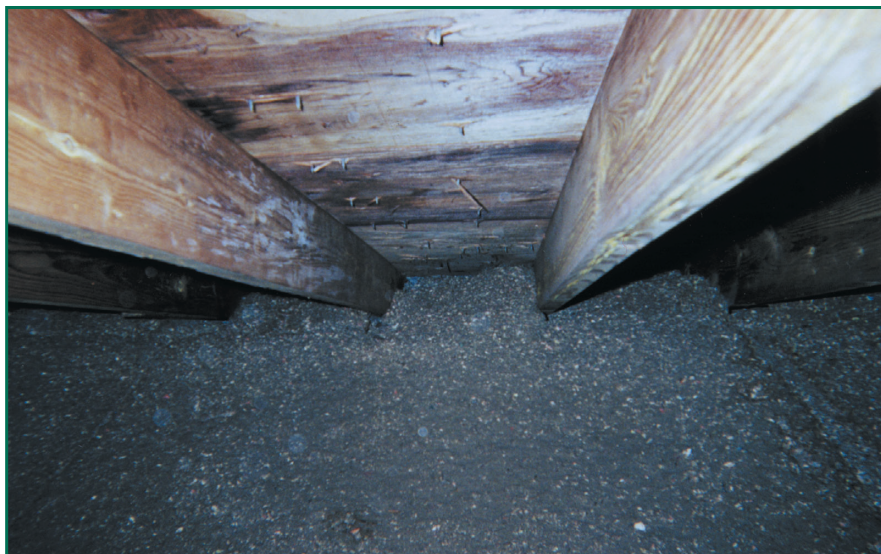
Figure 2: Fungus and spores and mold — Oh my! Mold/mildew accumulation in a humid southern attic. The colonies were fostered from a wintertime condensation scenario, drying during the hot season to the formation shown. Note that attic insulation must be held back in order for the soffit to serve as the intake port. A pre-manufactured baffle can be used to keep blown-in insulation from becoming a ventilation impediment.
