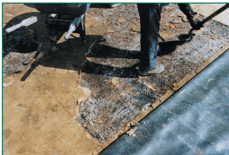
Figure 3: Fungal colonies found during a roof tear-off. Colonies had spread widely below the roof covering. When entrapped water reaches the building interior, the same fungal colonies can grow on roof decks and framing members.
