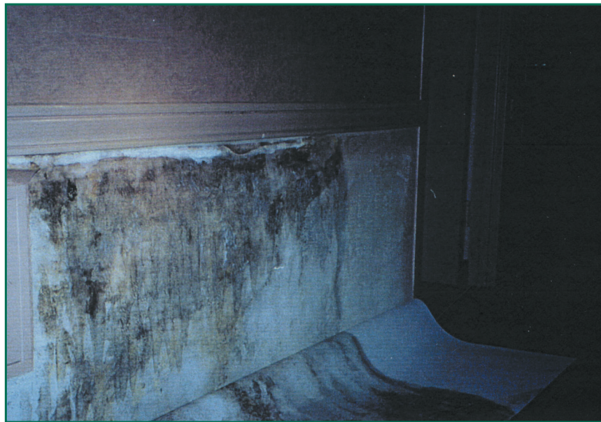
Figure 6: Severe accumulation of mold colonies, thriving on the paper facing of the gypsum drywall and kept wet by the low permeability of the vinyl-backed wall covering. The condition is unrelated to a single identifiable storm event.
