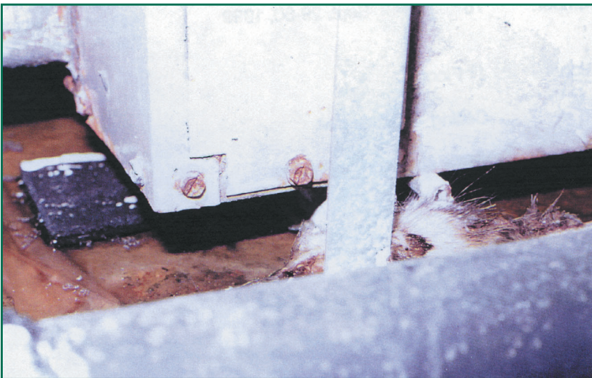
Figure 5: A condensate pan beneath an HVAC unit. Not only was a curious mix of molds being fostered, a dead rat was floating in the water. The condition was found in several other rooms of this upscale hotel.
