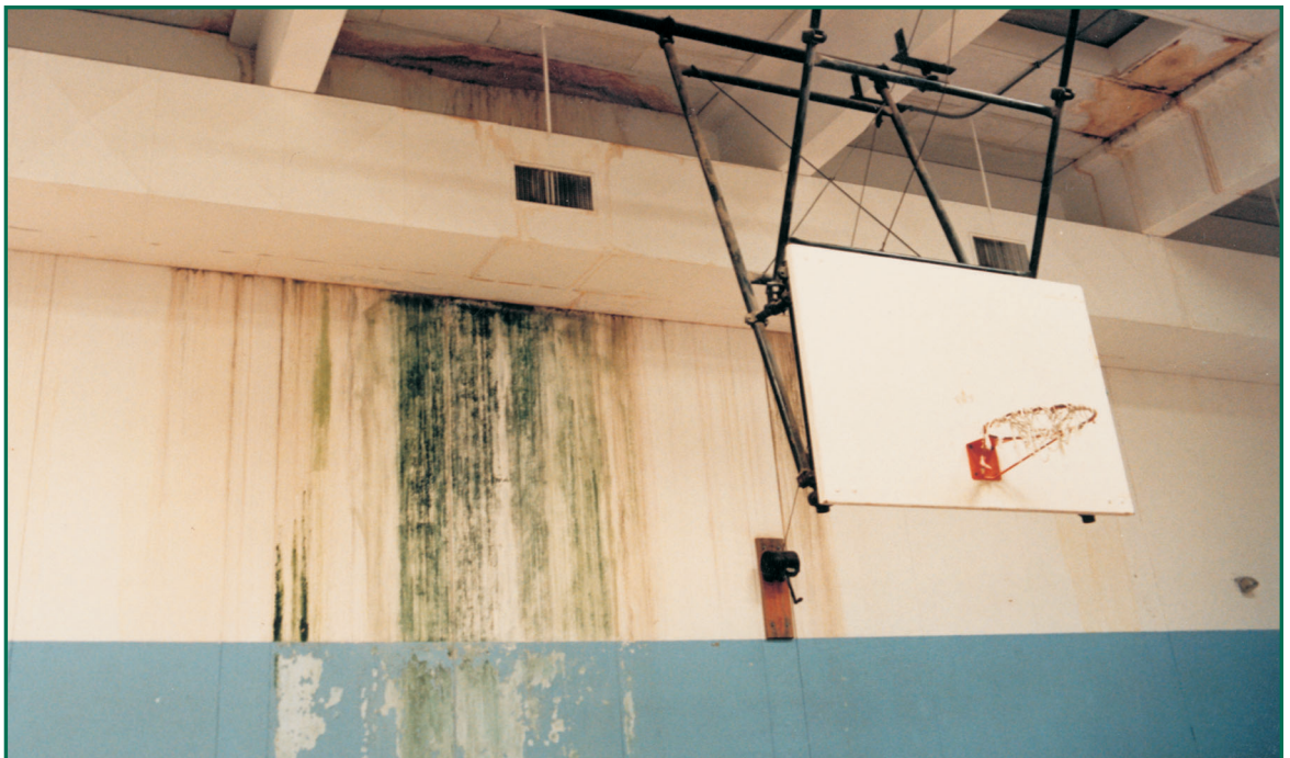
Obvious damage has been done by moisture and mold in this gymnasium.
