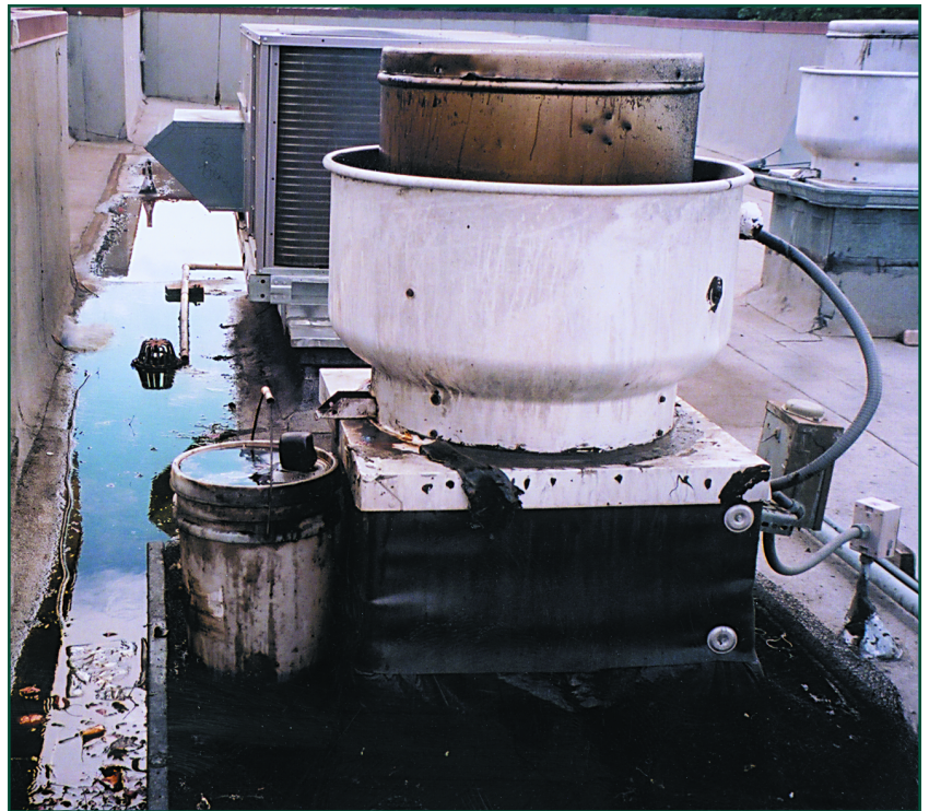
Photo 1: Grease spilling from a typical rooftop exhaust fan that does not have proper grease containment product in place.
