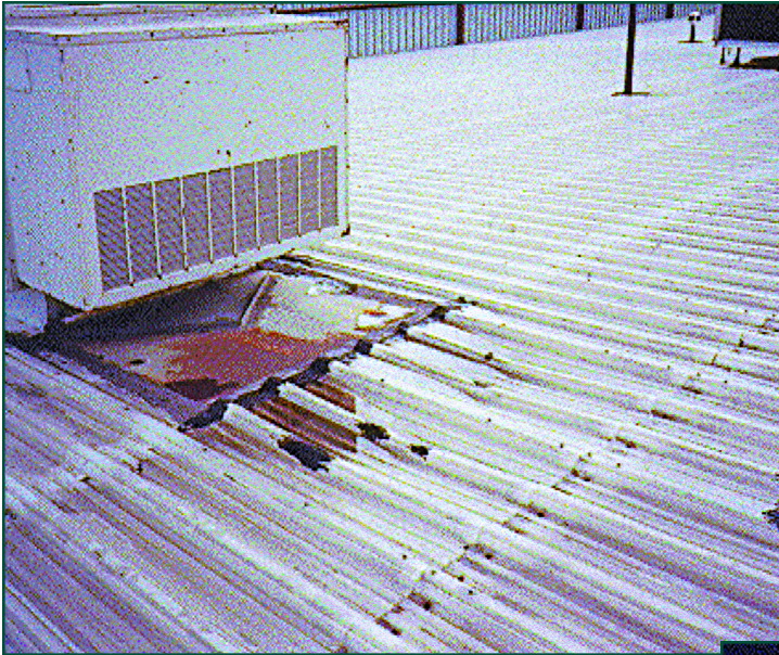
Figure 5 — Curb penetration has exposed screws and ponded water.
