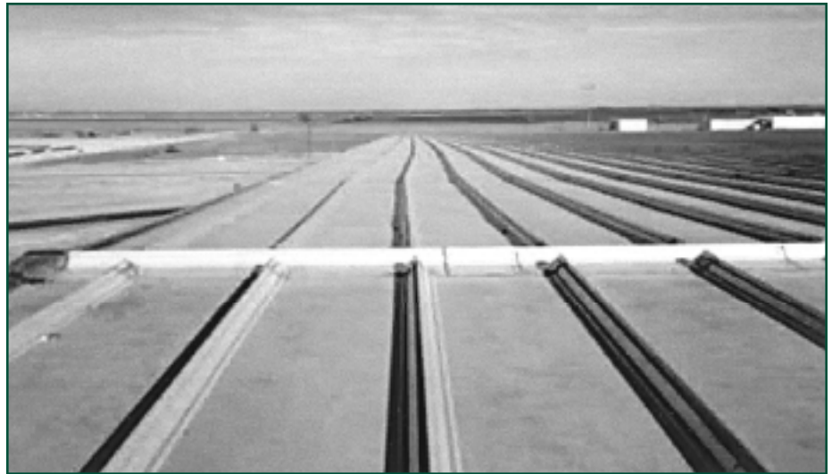
Figure 8 — A standing seam roof that has been installed out-of-module and also has been misaligned as evidenced by the changes in direction of the panel seam.
