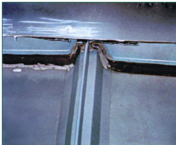
Figure 3 — Poor panel alignment leads to poor fit-up of the panel closure.
