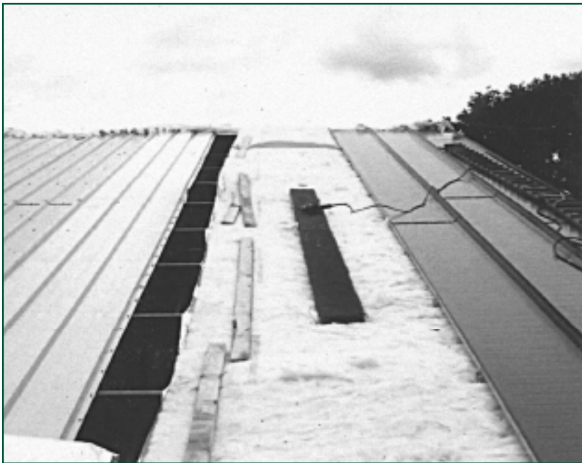
Figure 11 — A new standing seam roof (dark-colored panel) being installed from the right.
