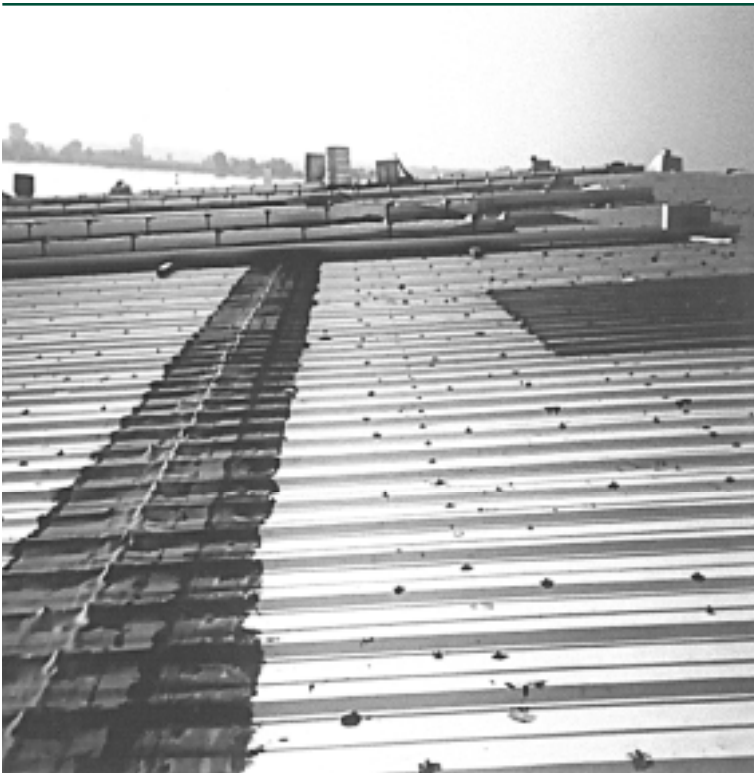
Figure 12 — An attempted fix using asphalt-based products that must be fully removed before application of an elastomeric type coating.
