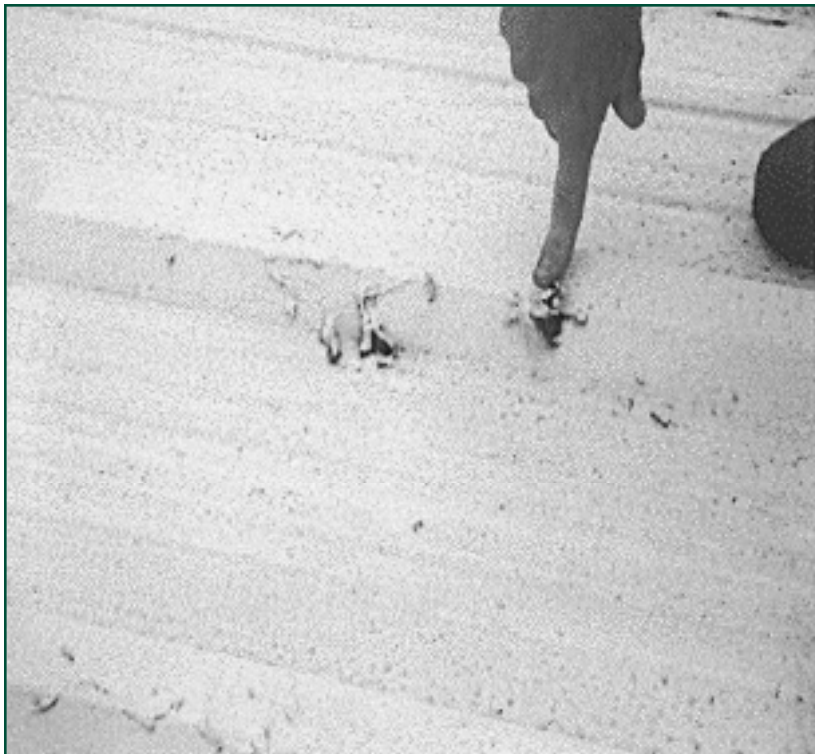
Figure 13 — Failure (bleed-through of underlying material) of an elastomeric coating due to improper surface preparation.
