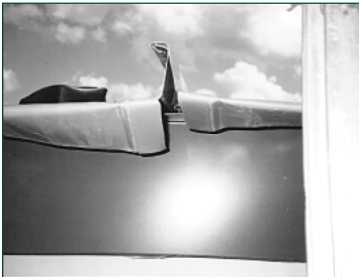
Figure 6 — Close-up view of open, unsealed metal roofing panel edges at eave/gutter and wall connections. This is a total waterproofing failure.
