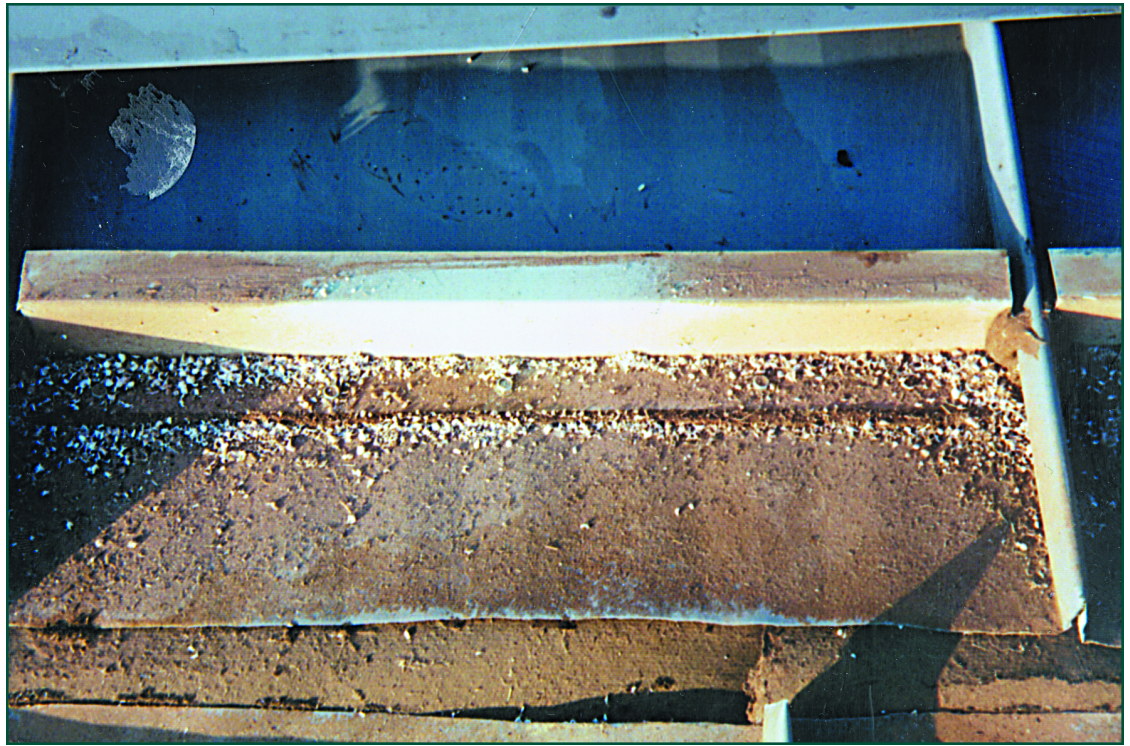
Figure 2 — Close-up view of the metal roofing panel and closure and ridge cap flashing. Water and debris stains are clearly visible. Areas showing debris are supposed to be watertight.
